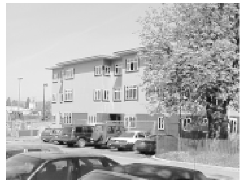
A graduate housing project underway on the campus will help to maximize housing options within walking and biking distance for students.
