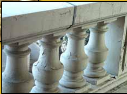
*Restoration: stonework damaged by earthquakes
