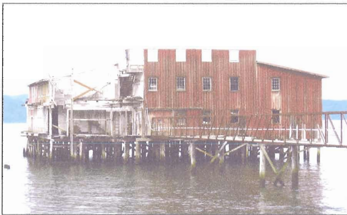
Figure 25. Union Coop net warehouse, “Big Red.” Damaged by storm in 2004. Source: Author
