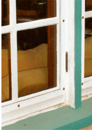
Figure 5 – Detail of exterior of restored living room casement window showing the unobtrusive wood-framed exterior storms directly mounted on the frame of the window. Restored original hinge is visible as well.
