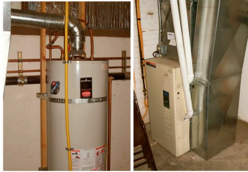
Figures 7/8 – New high capacity water heater, anchored to the basement wall per latest codes. High efficiency furnace uses plastic pipe for exhaust gases.
