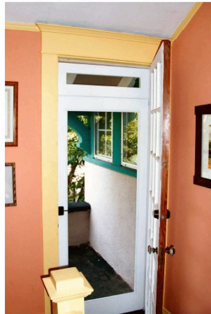
Figure 6 – Wood-framed storm/screen door replaced non-compatible aluminum storm door at the second floor balcony door. Wood framed glass storm insert can be attached with simple metal clips.
