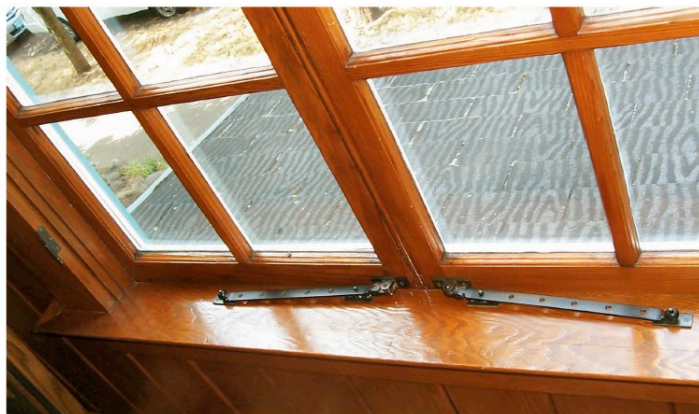
Figure 4 – Detail showing restored casement window in dining room, with closer bars found in basement.
