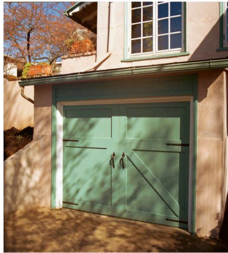
Figure 3 – New garage door. This is a standard overhead door with modern track and opener mechanism, but with Craftsman Style carriage house door appearance. Per approval by SHPO from contractor's working drawings.
