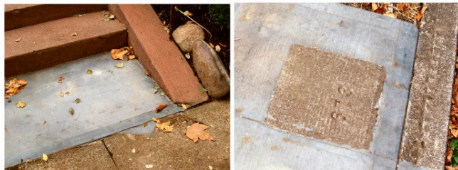
Figures 11/12 – Two views of city-mandated sidewalk repairs. On the left is the portion of the original red concrete replaced to meet city codes. On the right, a portion of the walk going to the curb (covered by city codes due to its contact with the curb), replaced but with the “673” original house number cut out of the old concrete and reinstalled in the new.
