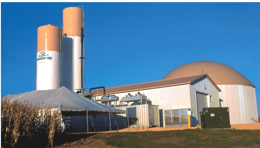
Figure 4. Complete mix digester
