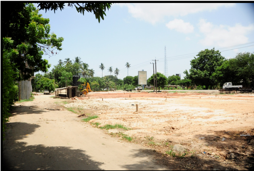
Figure 6.24. Paving over Drive In Farm. View from the opposite side of the farm. The truck in the left background sits in front of the building. The area that has been graded for paving consists of about half of the Drive In farm (A. Halloran).
