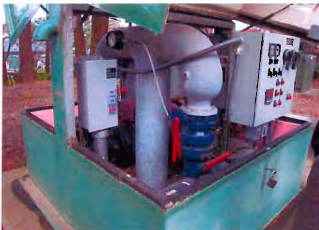
Figure 3-2. CRW Intertie Pumping Station
