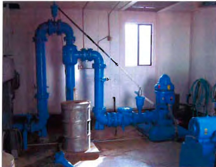
Figure 3-3. Well No. 2, Typical Well Discharge Configuration
