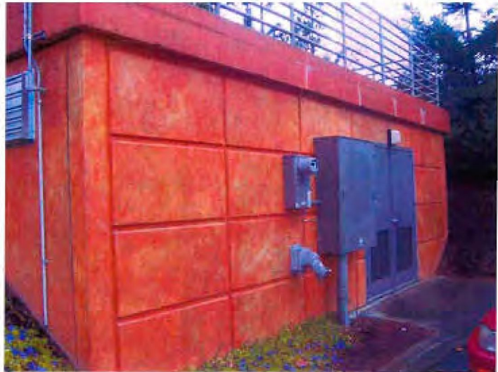
Figure 3-9. Lava Drive Pump Station
