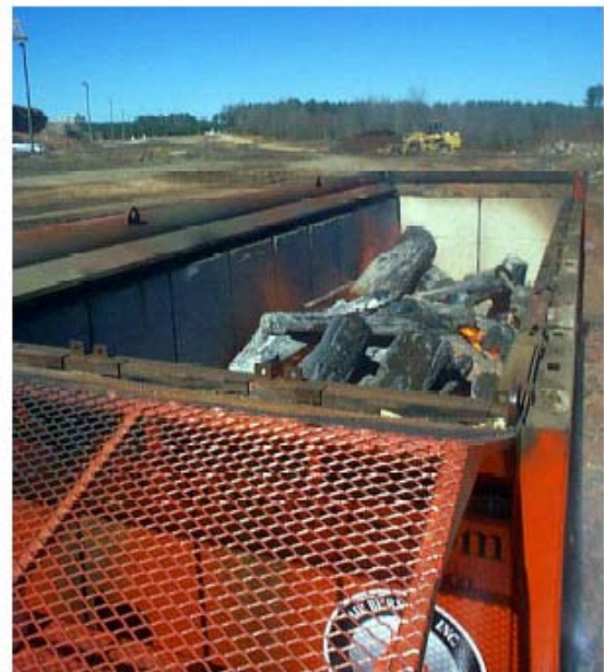
Figure 1—Skid mounted ACD in full operation (no visible smoke).
