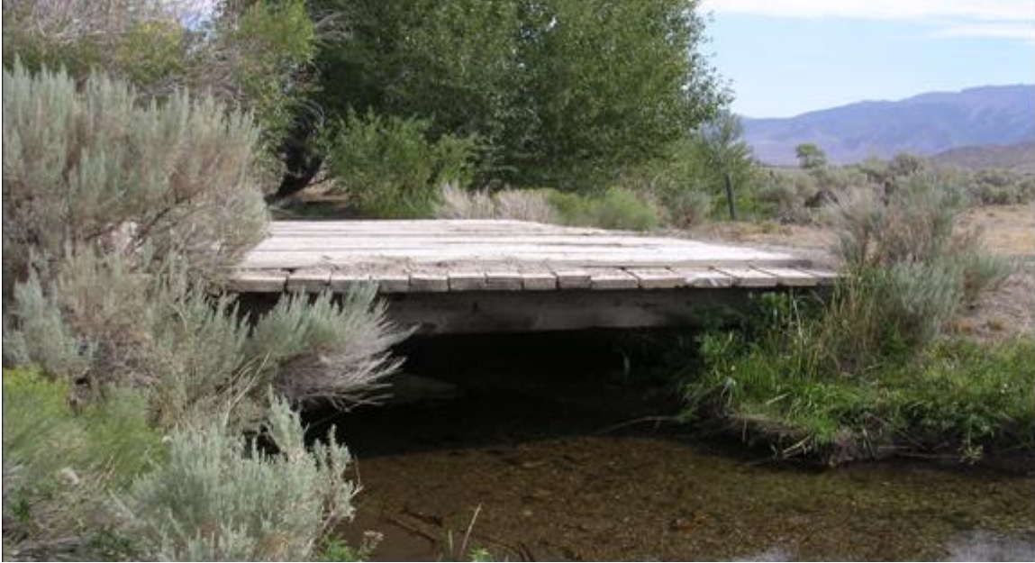
Figure 38. Potential dry hydrant located 4.0 miles southwest of Highway 93.
