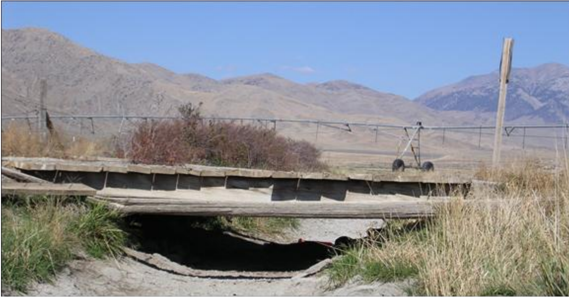
Figure 29. Limited capacity bridge. This four (4) ton weight limit bridge is located at 2400 North 2800 West intersection and one-mile north-northwest of Butte City.
