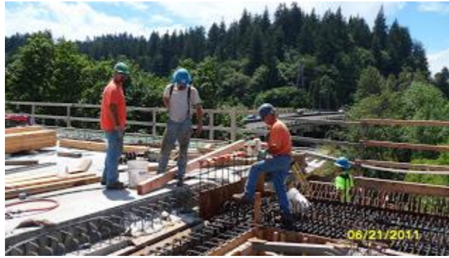
Crew members prepare to join a new section of bridge deck, at right, to one that was formed and poured earlier, at left.
