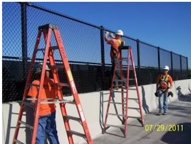
At the south end of the new Willamette River Bridge, special fencing on top of the concrete barrier protects the railroad tracks below.
