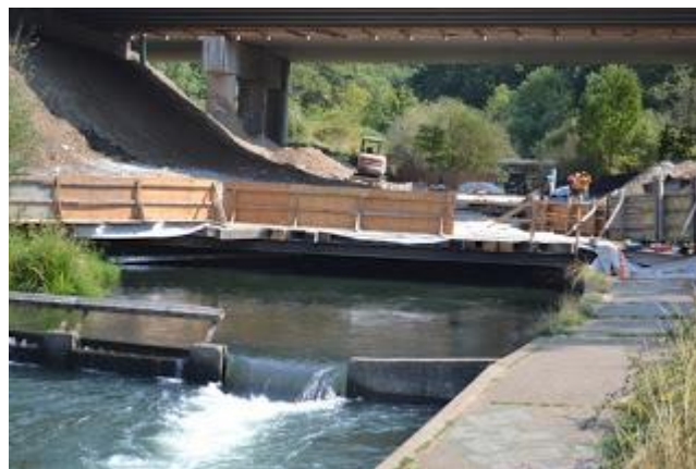
You can see how much of the walls have been removed so far.
