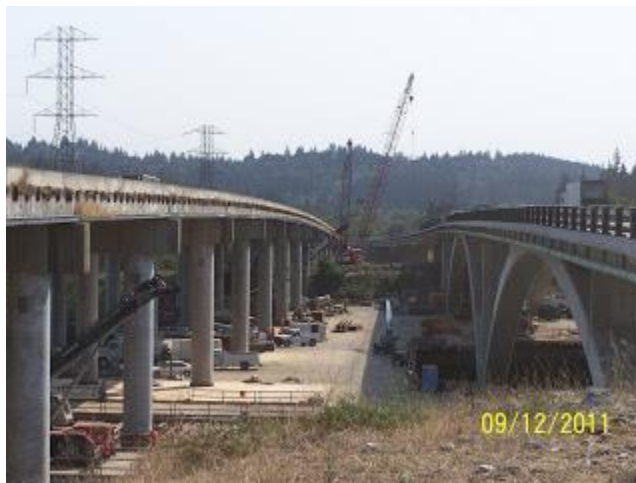
The graceful arches of new southbound Interstate 5 Willamette River Bridge right, stand in contrast to the long row of piers for the temporary detour bridge built in 2004.
