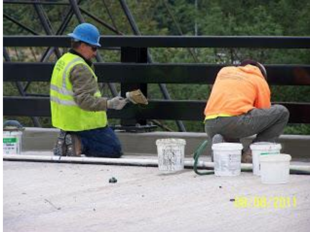
Workers put the finishing touch - shiny black paint - on the new railing.
