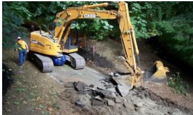
Crews tear up the old concrete path near Walnut Road to replace it with a soft path.
