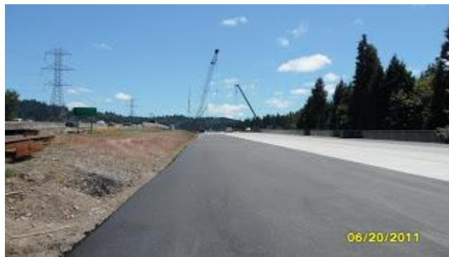
The newly paved asphalt shoulder contrasts sharply with the shiny white concrete of the southbound bridge. The cranes in the background mark where the main span crosses the river.
