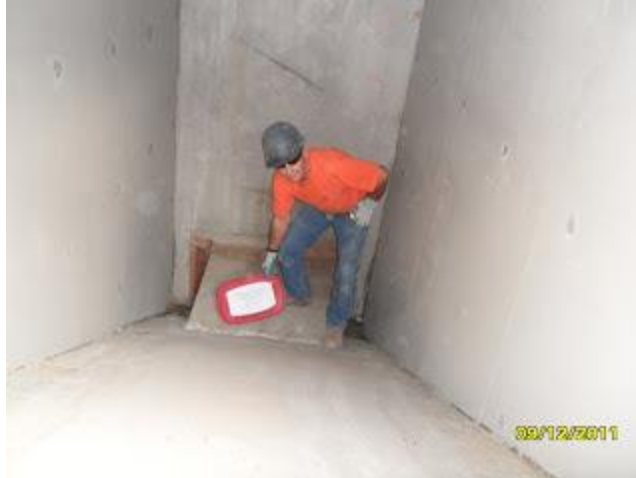
Bob Vaughn, Hamilton foreman, displays the time capsule, and then places it in the bridge arch.
