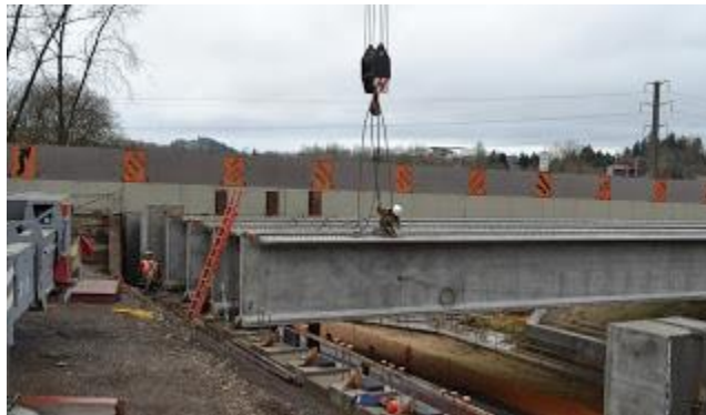
With the beam in place, workers disconnect the cables used for lifting the beam.
