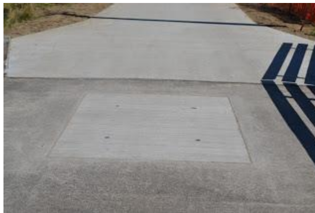
A new concrete lid on the north end of the Knickerbocker Bridge allows EWEB to more easily reach the water pipe
