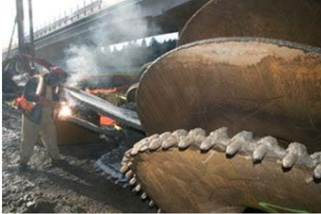
This worker standing next to the drill bit or auger illustrates just how large it is.
