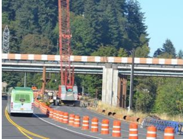
The final columns-- on the north side of Franklin Boulevard-- rise above the roadway along the south bank of the Willamette River.
