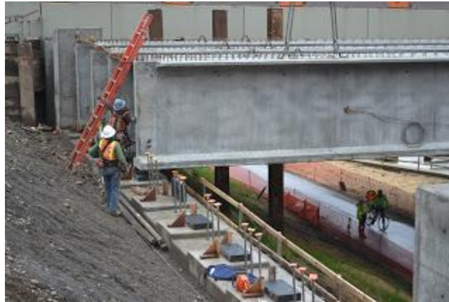
Flagger shown in the lower right corner is stopping a bicyclist until the beam is set into place.
