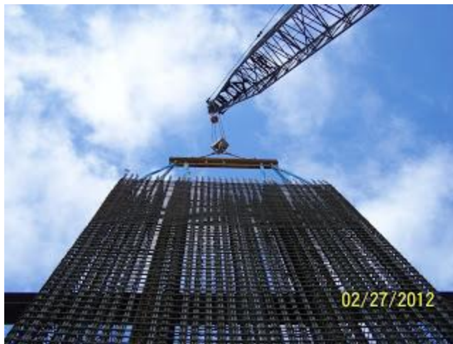
A large crane lowers the tied rebar down into a shaft to form an abutment wall.
