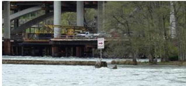
Upstream of the I-5 bridge construction work, a sign at the old dam structure directs river traffic to the safe channel on the right.
