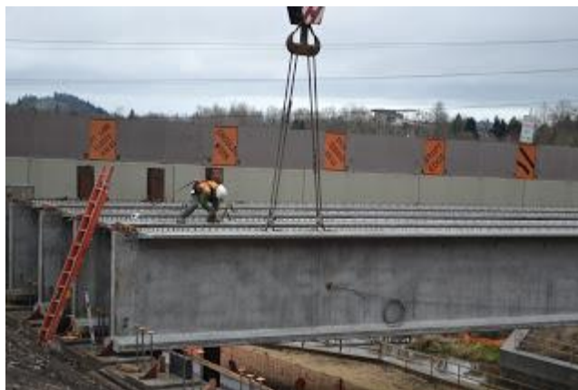
A worker is protected by a safety rope while he is on the beam.
