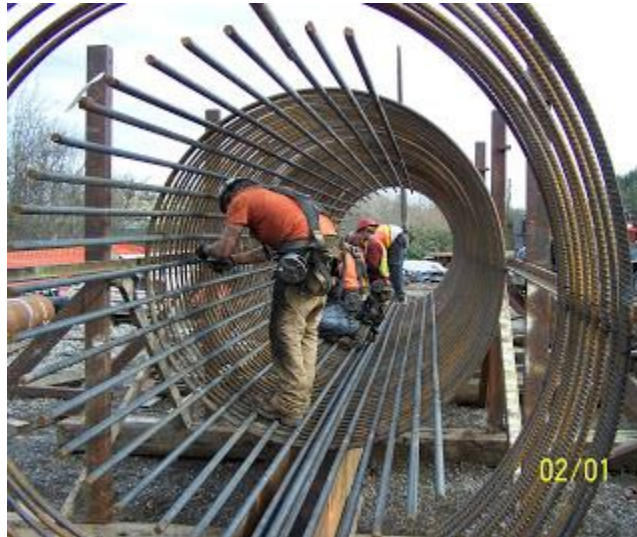
Ironworkers tie the steel rebar to form the pier cages in a work area in Alton Baker Park, just north of the Knickerbocker Bridge.
