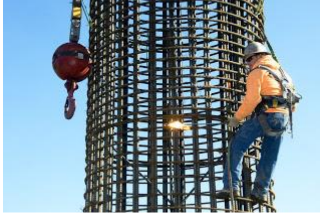
Ironworkers and welders build the steel structures by tying together miles of rebar.
