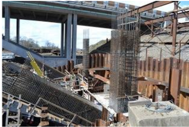
Workers build a column inside a cofferdam on the Willamette River's north bank.
