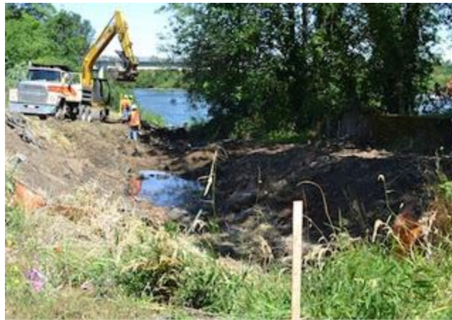
Workers are clearing out overgrowth and creating a new stream channel along the south bank of the Willamette River.
