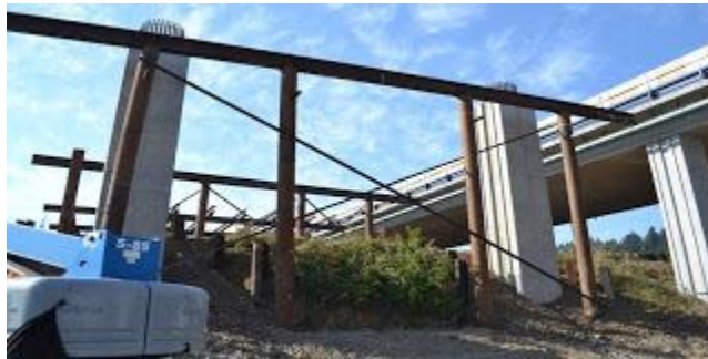
The columns shown from the riverside stand alongside steel structures built to support the bridge falsework. The exposed rebar on top will connect the columns to the bridge deck when it is poured.
