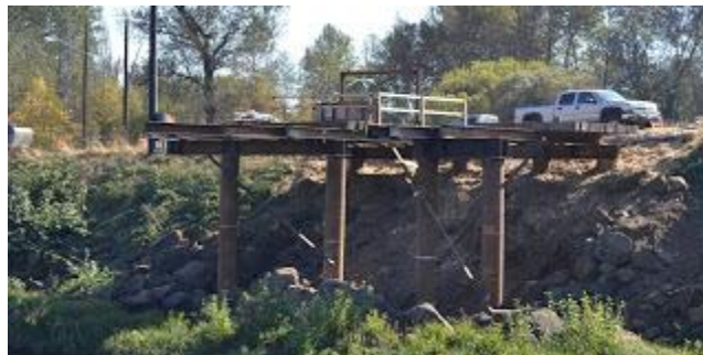
Here is one of 12 work platforms built on the riverbank to support heavy equipment.
