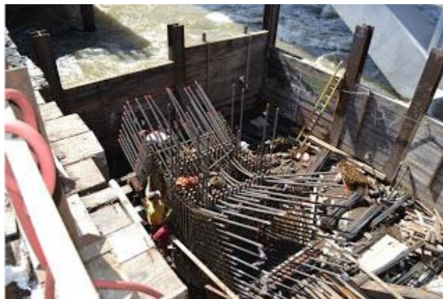
This cofferdam protects workers as they install rebar for bridge arches in the center of the river.
