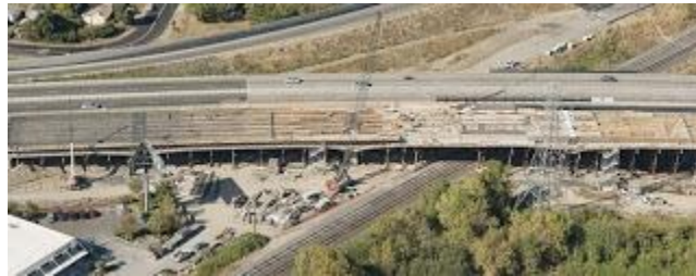
This picture, taken in November from upstream, shows the arches for the new northbound bridge under construction. The final concrete pours joining the arch sections will occur this month.
