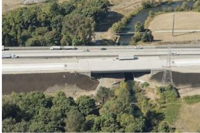
Construction of the new Canoe Canal span also began and completed in June.
