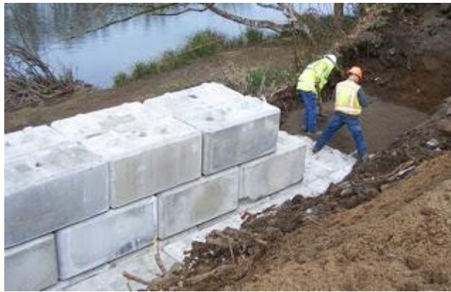
K & E Excavators shovel base rock to ensure the base is level.
