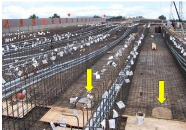
Here you can see part of the rebar skeleton that makes up the bridge beams. The arrows point to plugs that create the oval access holes when concrete is poured for the beams.
