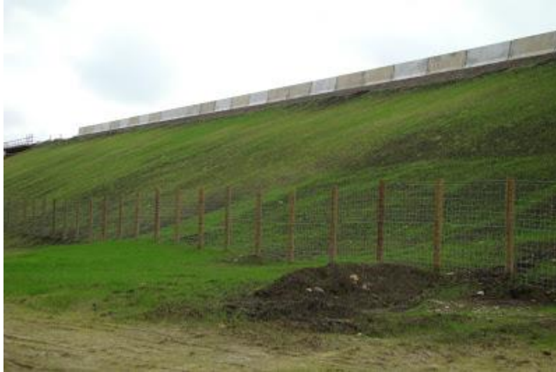
Grass seed matures on both sides of the new right of way fence installed on the east side of the new northbound I-5 bridge.
