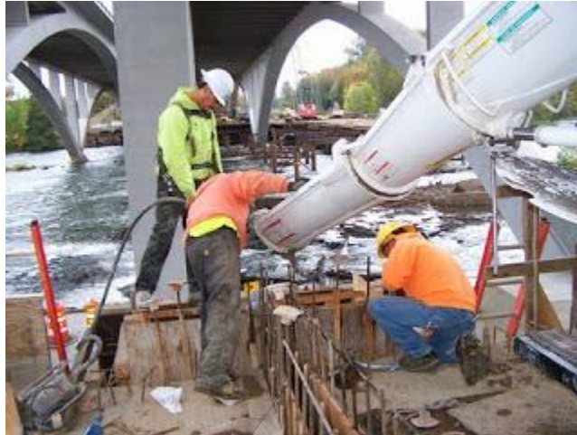
In this photo, crews are pouring concrete between the path beams to seal them together; this segment of the path passes by the base of the highway bridge arches.
