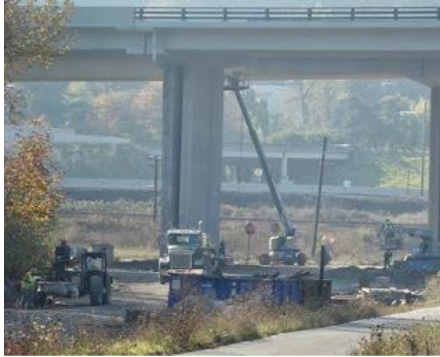
Crews use a manlift to finish details on the underside of the bridge.
