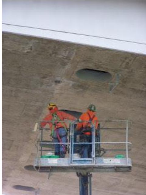
Workers get ready to enter one of the access holes to finish the interior surfaces of the bridge's concrete beams and decks.
