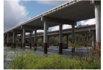
The I-5 Willamette River Bridge crosses the Willamette River in the Eugene-Springfield area.
