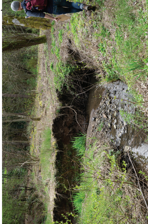
erosion west of 68th
