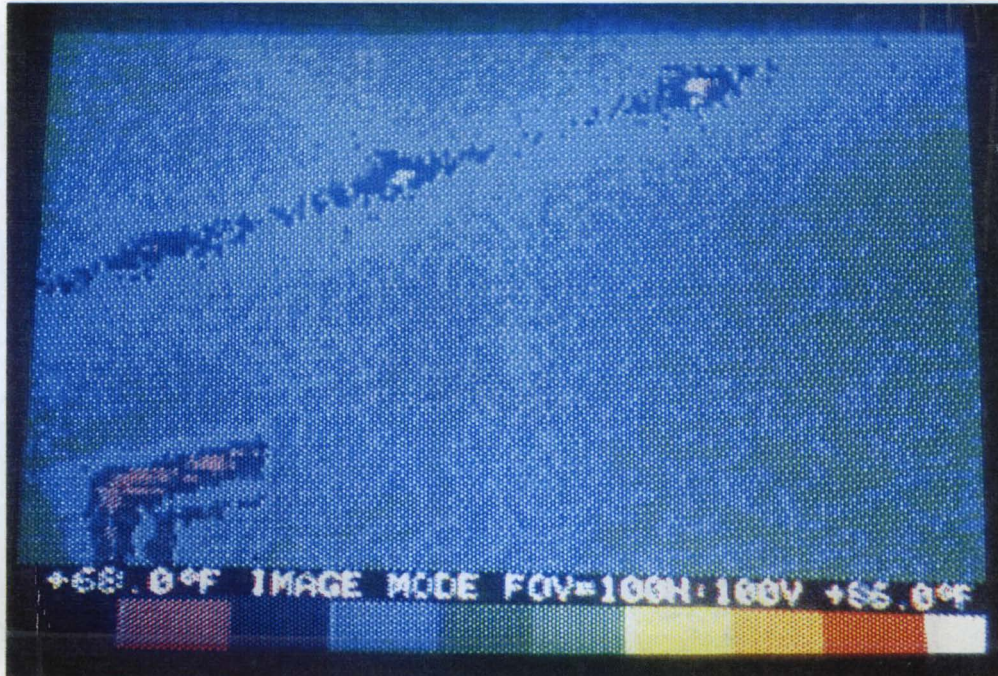
Figure 7.3-4 Heat loss at joint of wall and vaulted ceiling and at window. Heat loss at wall framing and roof truss framing more pronounced.
