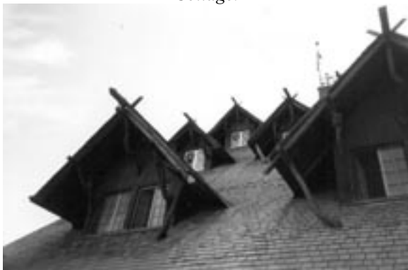
From our side trip...Dormers on the roof of the Old Faithful Inn, in Yellowstone National Park.
