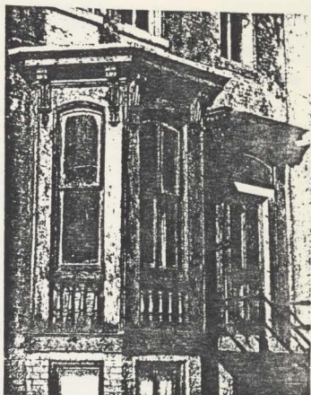
Fig. 2 A traditionally painted bay window has been stripped to bare wood, then varnished. In addition to being historically inaccurate, the varnish will break down faster as a result of the sun's ultraviolet rays than would primer and finish coats of paint. Photo: David W. Look, AIA.
