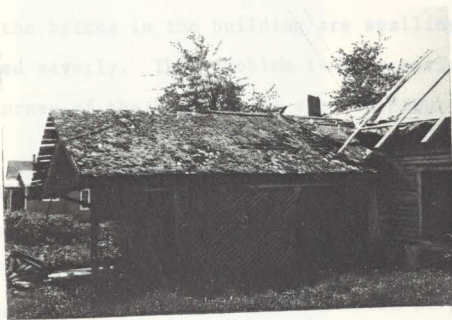
Fig. 35. View of north side of woodshed roof showing thick layer of moss.
