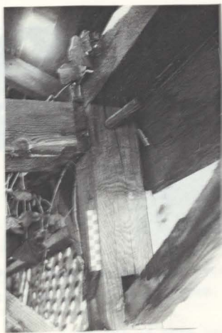
Fig. 32. Deteriorated mortise and tenon joint on the north side of the woodshed.
