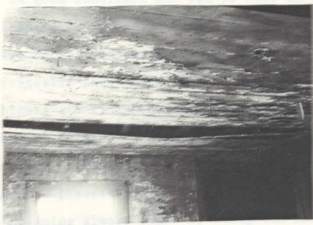
Fig. 28. Deteriorated ceiling boards on the west side of the kitchen ceiling.
