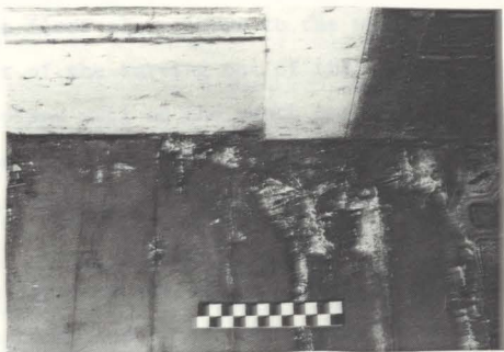
Fig. 23. Hyphae and white surface growth of a decay fungus along the east side of the kitchen floor. (scale = 6")
