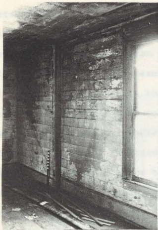
Fig. 4. West wall of the dining room, showing the transition from box to balloon construction.
