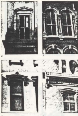
Illus. 5. The four historic examples of various window head-shots are: (a) stone, (b) cast stone, (c) cast iron, and (d) sheet metal. The criteria for selecting substitute materials (style, availability, quality, delivery dates, cost) are not much different from the past. Photo: Sharon C. Park, AIA.
