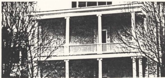
Columns were repaired and a capital was replaced in epoxy on this 19th-century 2-story porch. Photo: Dell Corporation
