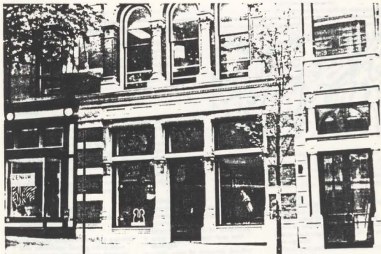
The new cast aluminum storefront replaced the lost 19th-century cast-iron original. Photo: Sharon C. Park, AIA.
