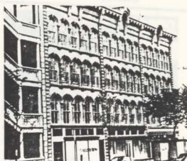
Illus. 22. A fiber reinforced polymer (fibreglass) concrete and precast concrete elements replaced deteriorated features on the 19th-century exterior. Photo: Sharon C. Park, AIA.
