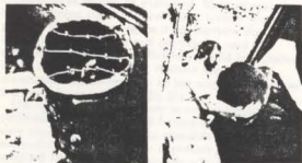
Illus. 17. Care must be taken to ensure that the replacement materials will work within a pre-designed system. At the Norris Museum, Yellowstone National Park, the 12-inch diameter log rafters, part of an intricate truss system, had rotted at the inner core from the exposed ends back to a depth of 48 inches. The exterior wooden shells remained intact. Fiberglass rods (left photo) and specially formulated structural epoxy were used to fill the cleaned out cores and a cast epoxy water end with all the detail of the original wood graining was laminated onto the log end (right photo). This treatment preserved the original feature with a combination of repair and replacement using substitute materials as part of a well thought out system. Photos: Courtesy of Harrison Goodall.
