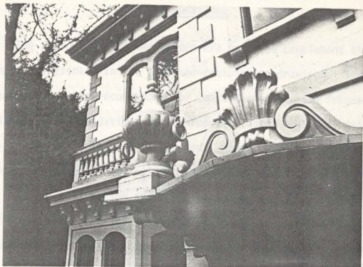
FIGURE 32. Glass Fiber-Reinforced Polymer Finial on the Kamm House in Portland, Oregon: 1988 View
