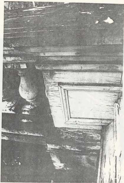
PHOTOGRAPH 1. Detail of Existing Engaged Pedestal on the North-Elevation Roof-Line Balustrade: Remodeled Circa 1949 (Note historically inaccurate flat-moulding profiles and the use of plywood.)
