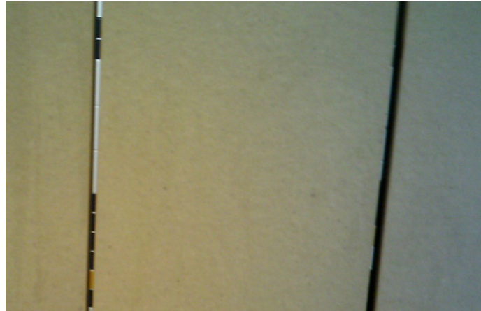
Figure 13: the gap in the stall door, as seen in a participant photograph.
