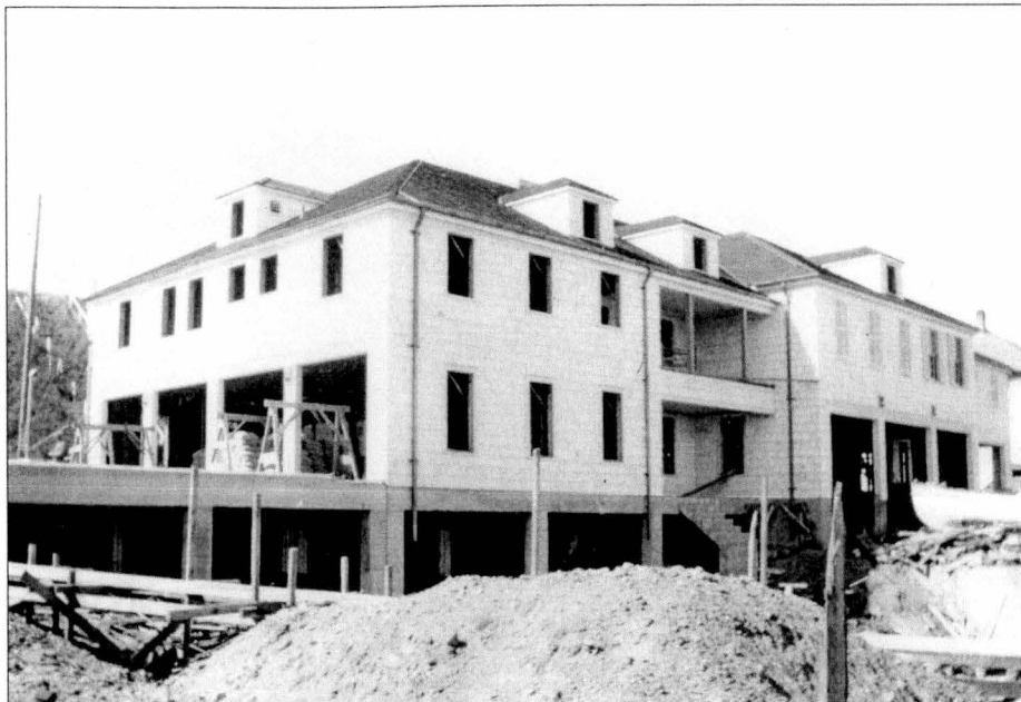
Figure 96. Coquille River Lifeboat Station Under Construction, 1939. Source: U.S. Coast Guard Headquarters (Coquille River File).
