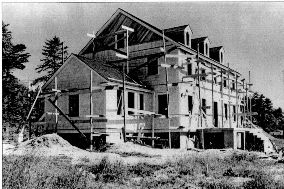
Figure 137. Yaquina Bay Station Under Construction, 1949. Source: U.S. Coast Guard Headquarters (Yaquina Bay File).
