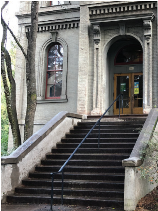
Metal stair railing is not original
