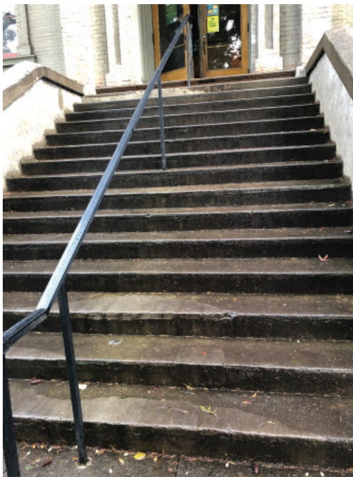
Stair treads are wider than at West Entrance, historically this entrance was designated for women
