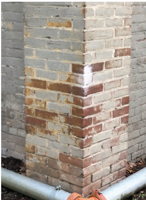
Exterior finishes deteriorating around northeast corner
