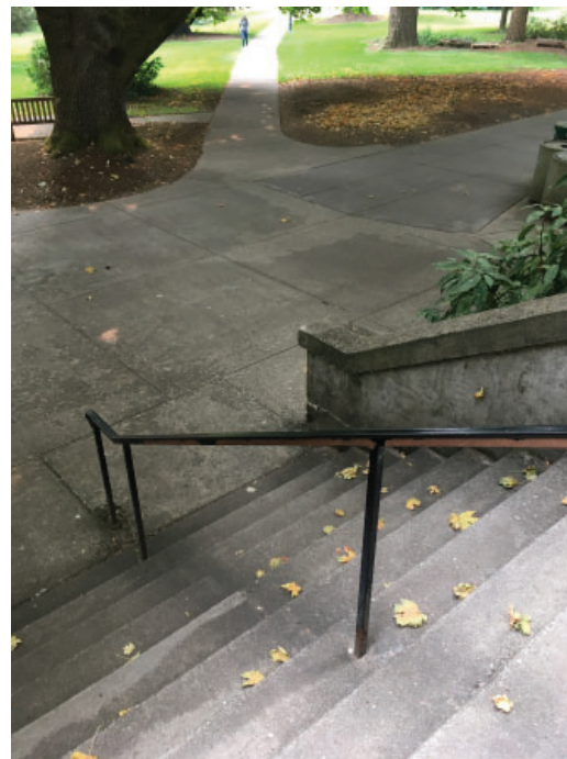
Single central rail is not original; design of concrete cap along the wing walls have changed over time
