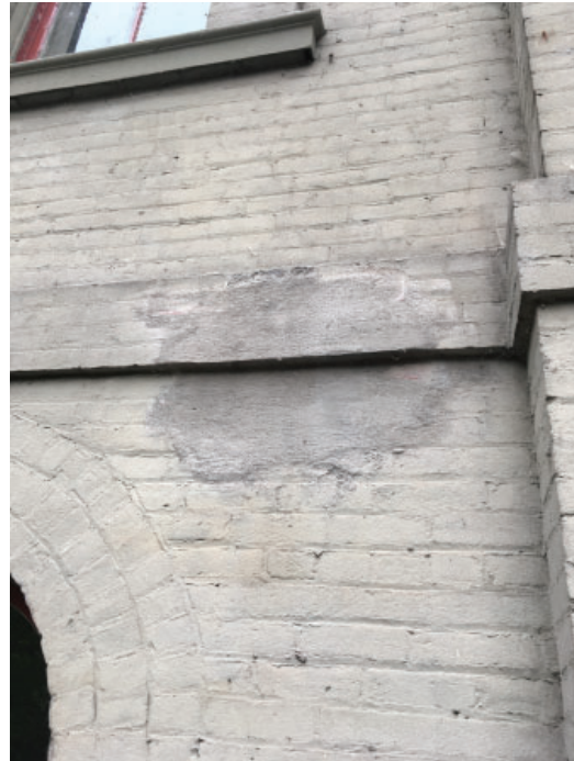
Prior repairs of infill brick do not match original color, texture or composition
