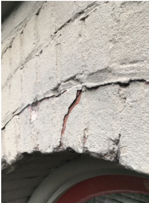
Finishes deteriorating around entryway
