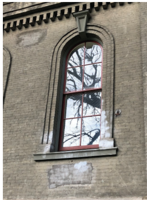
Previous brick repair does not match original facade
