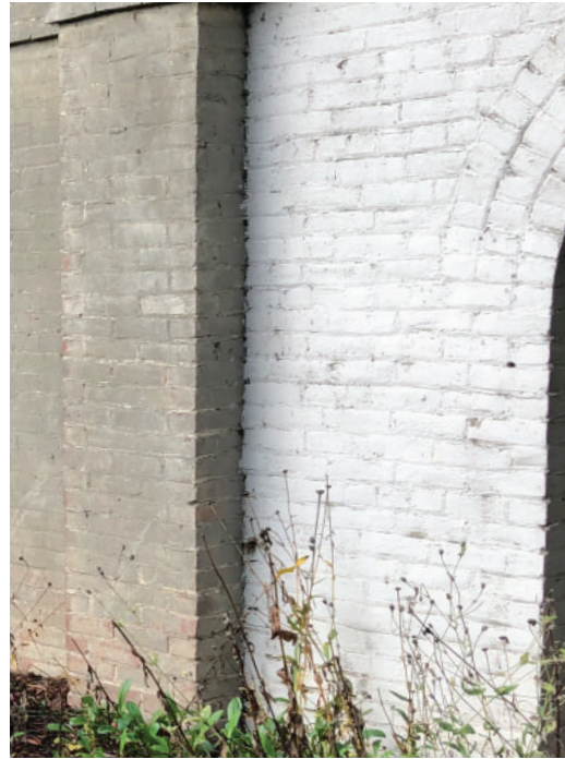
Facade finishes on southeast corner are different, brick was painted a different color
