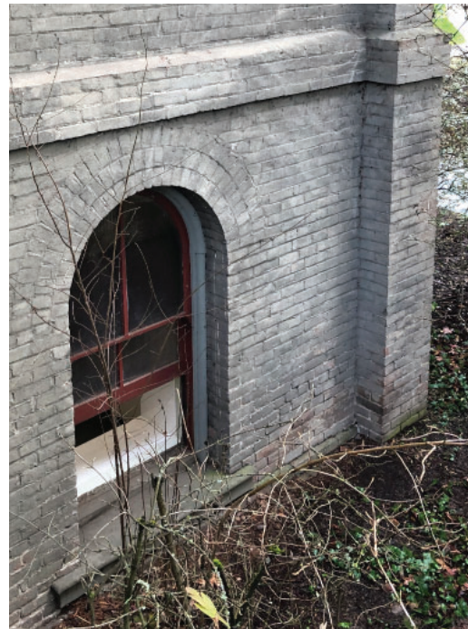
Facade finishes are deteriorating where facade meets the ground.
