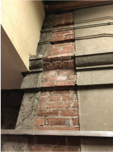
Some of the original west facade details remain, as viewed from the interior of the Robinson Theater. The west facade of Villard has stayed intact and are visible in some areas.
