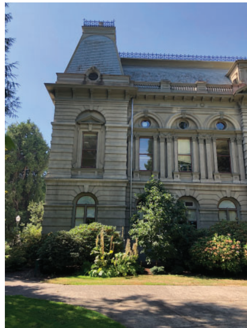
Missing decorative pediment (left), missing decorative urn details, and painted cedar roof shingles to mimic slate (paint is degrading on some more than others; replaced in kind during restoration).
