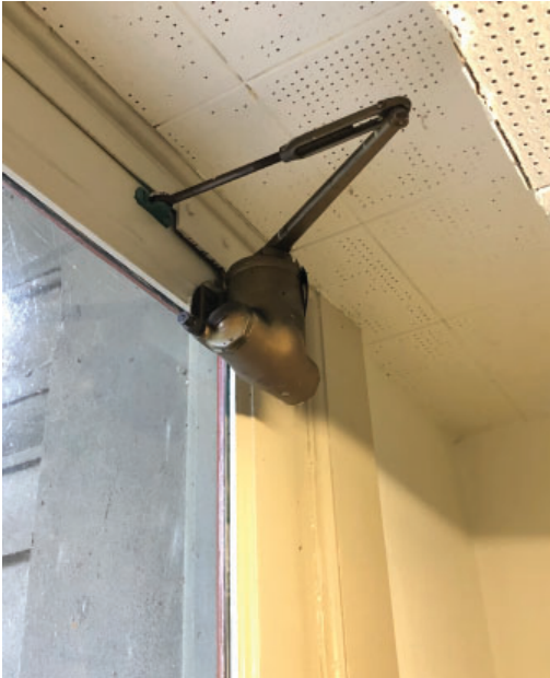
Older hardware on entrance door. (Further research needed to determine if these are original).
