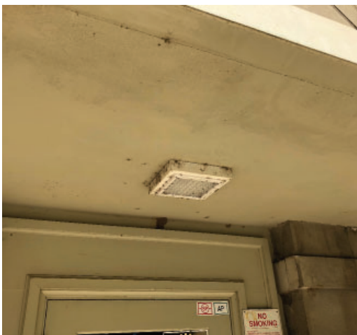
Incompatible light fixture.
