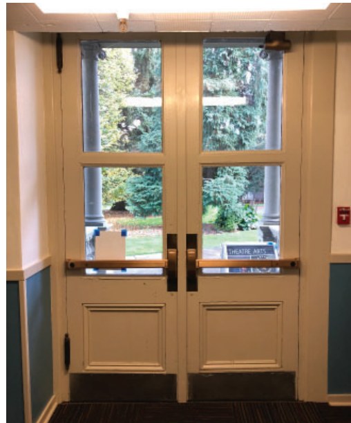
Newer hardware on interior of entrance. Added push open bar door handles on interior.
