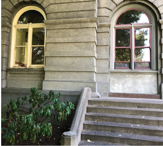
Different window trim paint colors, concrete wall infill at base of window (right).
