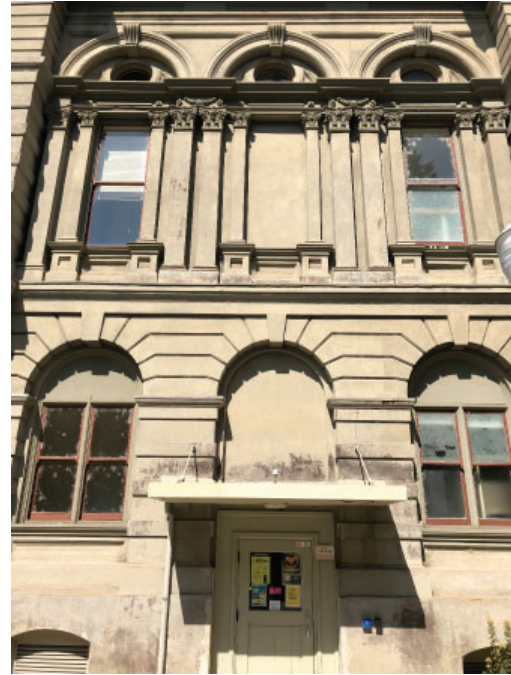
Missing second story window, center.
