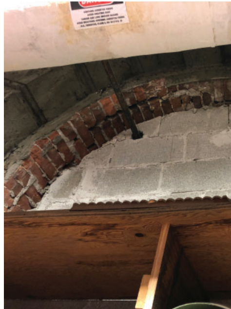
Archway infilled, utilities punch through wall to access Villard.
