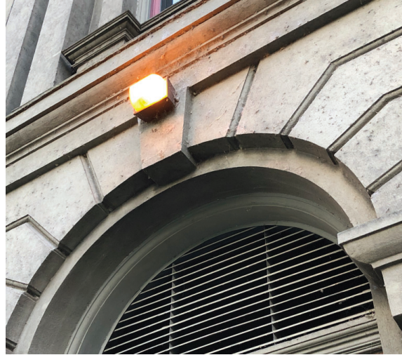
Incompatible light fixture over door.
