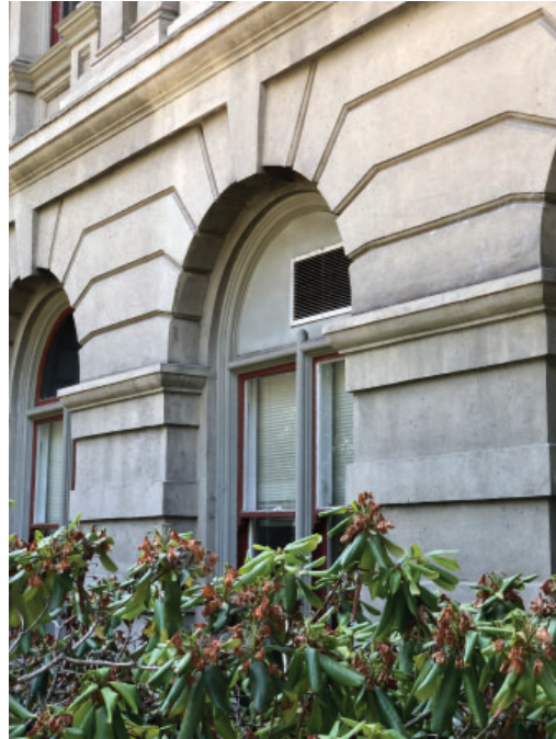
Incompatible air intake vent and missing window.
