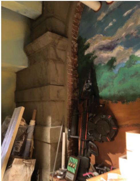
Archway infilled, mural painted in center, as viewed from the interior of the Robinson Theater. Utilities punch through wall to access Villard.
