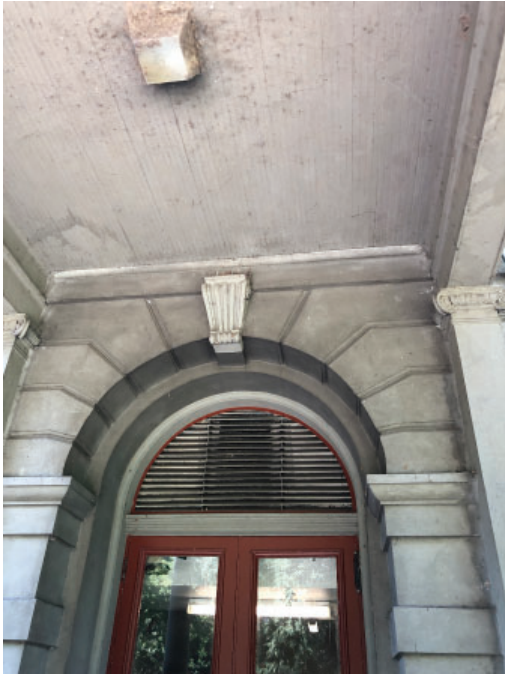
Incompatible light fixture and air intake vent.
