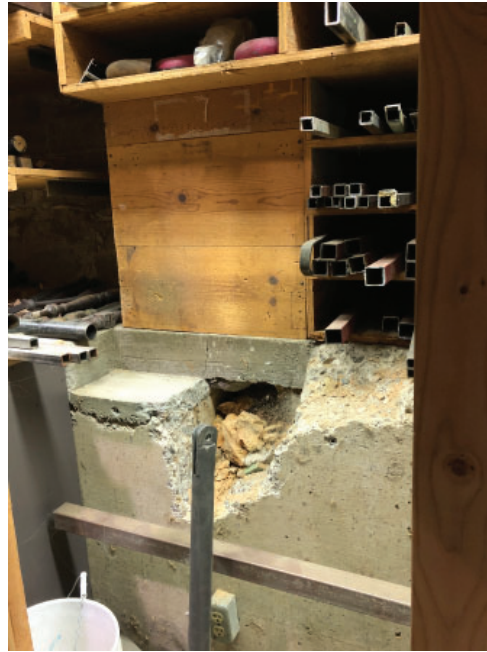
Foundation additions/changes on west facade, as viewed from the interior of the Robinson Theater.
