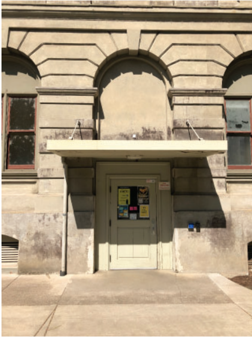
Missing window (center), incompatible overhang, entrance elevation, basement door removed, new doorway.
