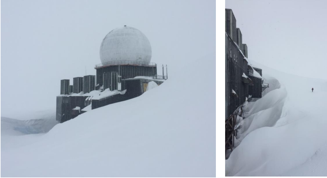
Figure 7 & 8: A recent visit to DYE-2 showing partial burial by snow (left). DYE-2 with adjacent figure demonstrating scale of building (right). Photo Credit: C. Max Stevens, 2017.
