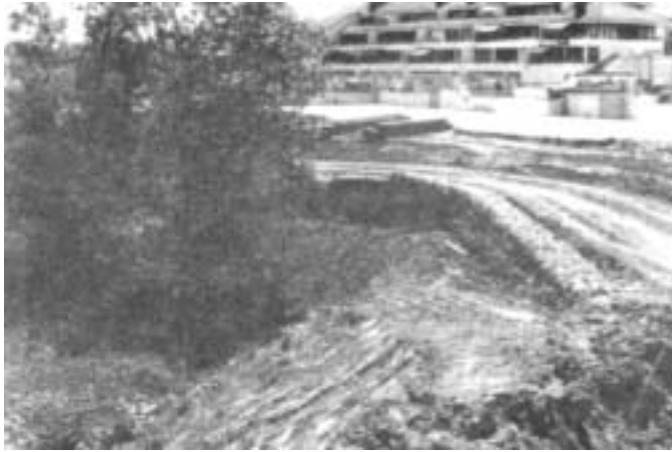
Designing the Greenway Trail and bank protection to go around smaller habitat areas helps to ensure their preservation. The trail and bank protection is under construction in this photo.
