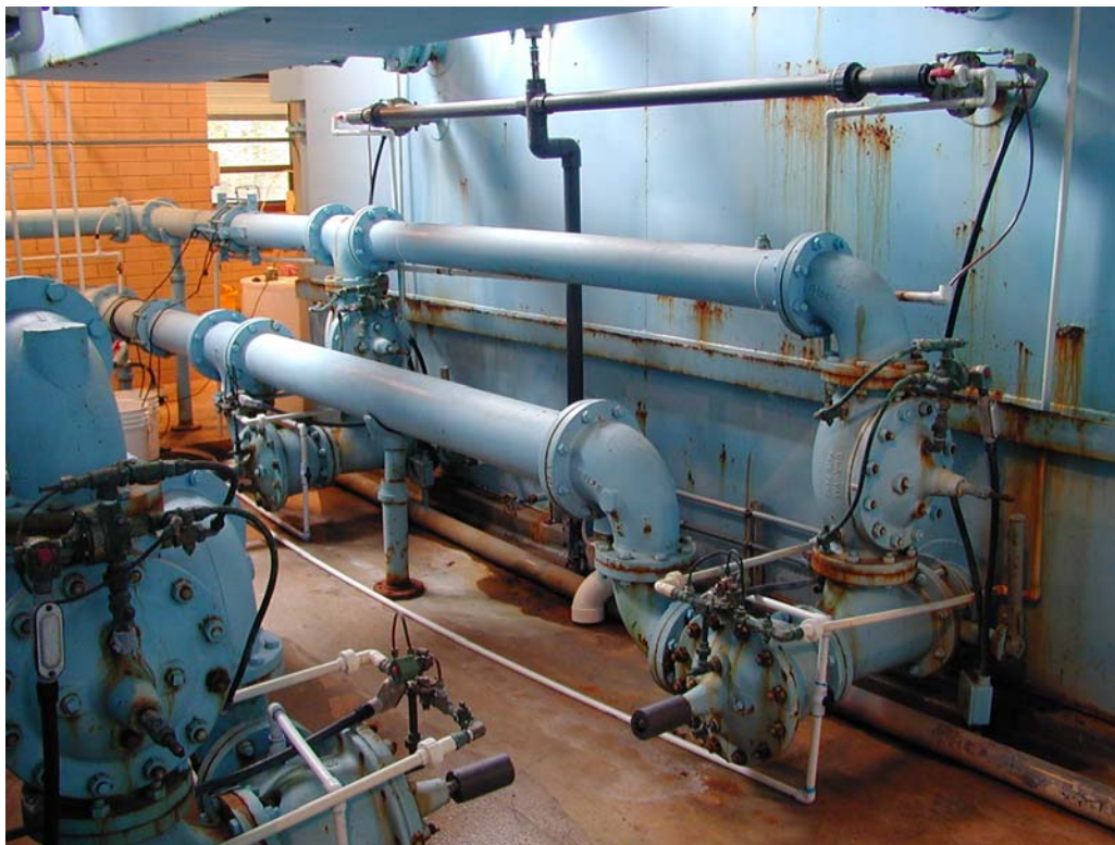
FIGURE 5.3.7 COOPER CREEK WTP FILTER UNIT & PIPING
