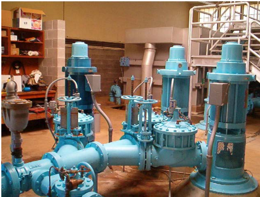
FIGURE 5.3.3 NONPAREIL WTP TREATED WATER PUMPS
