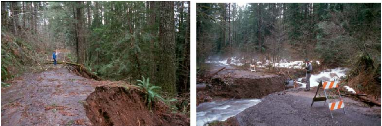
Figure 3.10. Example of catastrophic fill and culvert failure from the Mt. Hood National Forest Roads Analysis
