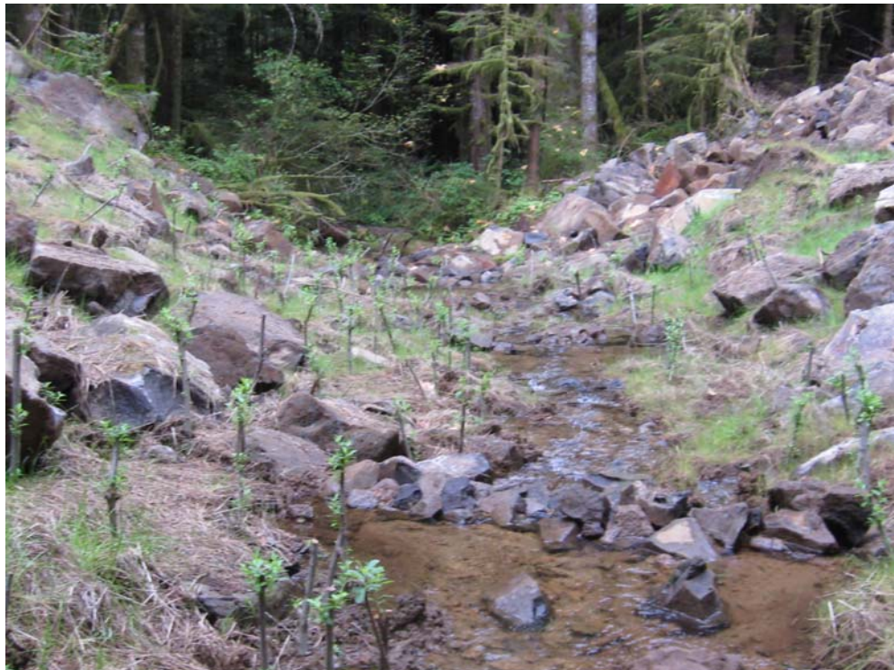
A Forest Service road once crossed this stream located on the Mt. Hood National Forest. The road was recently decommissioned restoring the stream to a natural condition and reducing the risk associated with the large fill located at this site.
