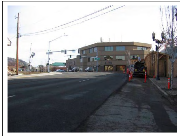
Greenwood Avenue @ Bond Street: Looking east into intersection from south side of Greenwood Avenue. bend 122.jpg
