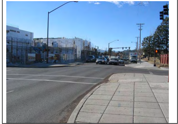
Arizona Avenue @ Bond Street: Looking west along north side of Arizona Avenue. bend 046.jpg
