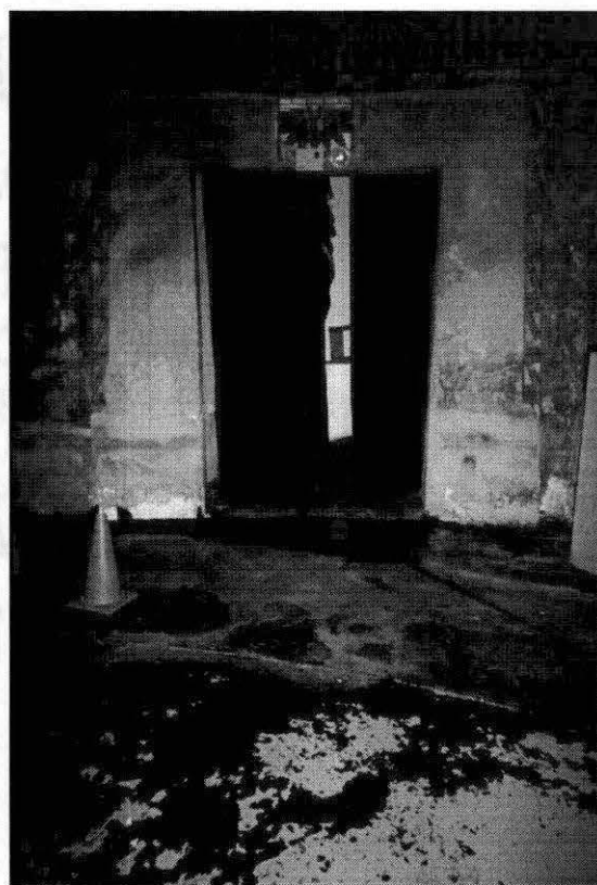
Figure 38. Wet Floor in Front of Exit, Egyptian Theatre, Coos Bay. Photo by Author, May 1998.
