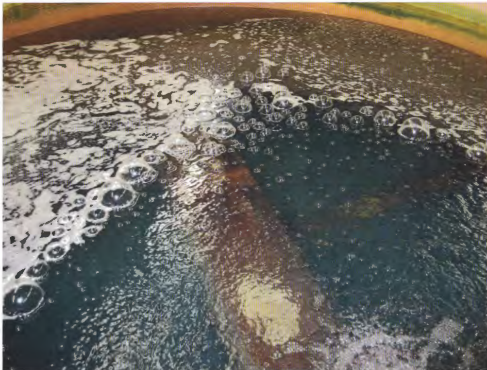
FIGURE 5.3.6 TOP OF FLOCCULATION BASIN
