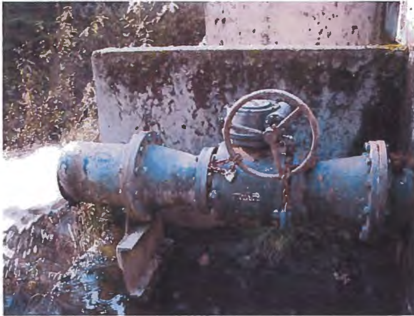
Outlet control valve
