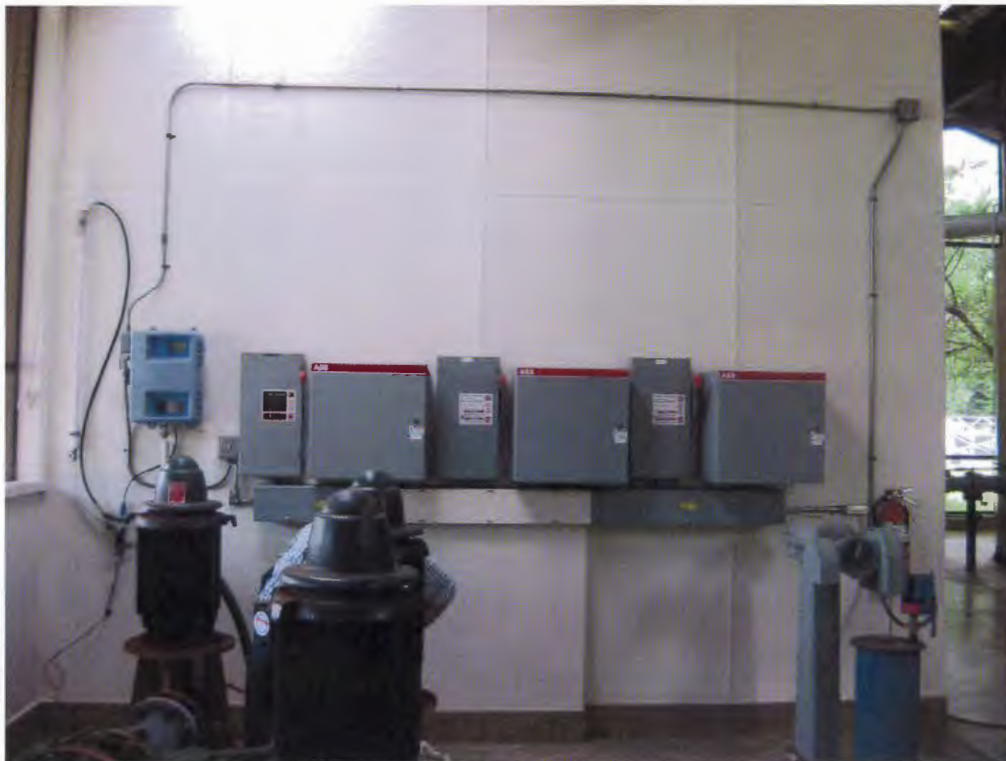
FIGURE 5.3.12 TREATED WATER PUMP AND LEVEL CONTROL SYSTEM
