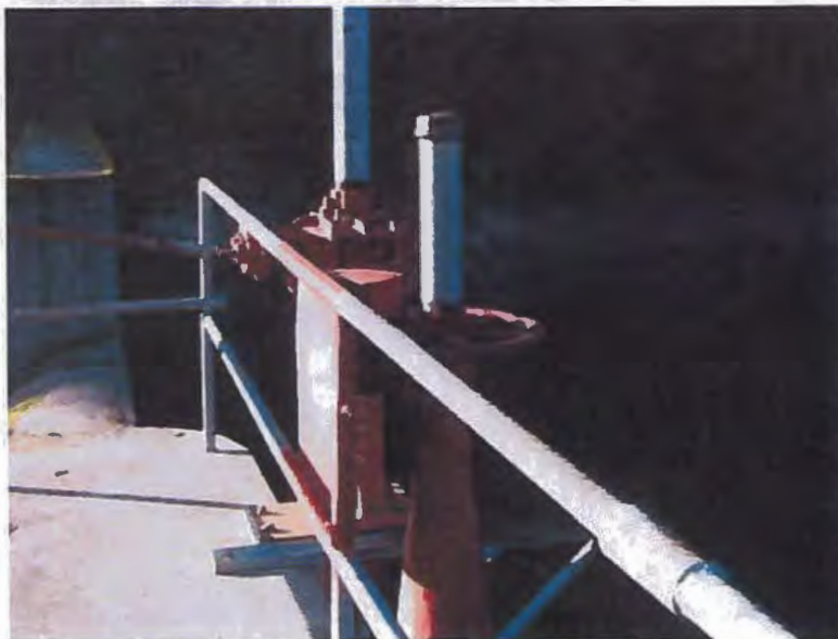
Control for valve and sluice gate
