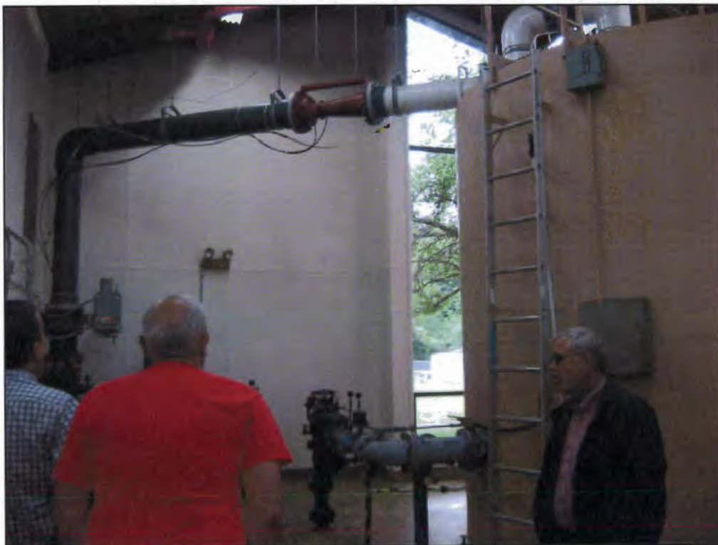
FIGURE 5.3.4 RAW WATER FEED TO FLOCCULATION TANK
