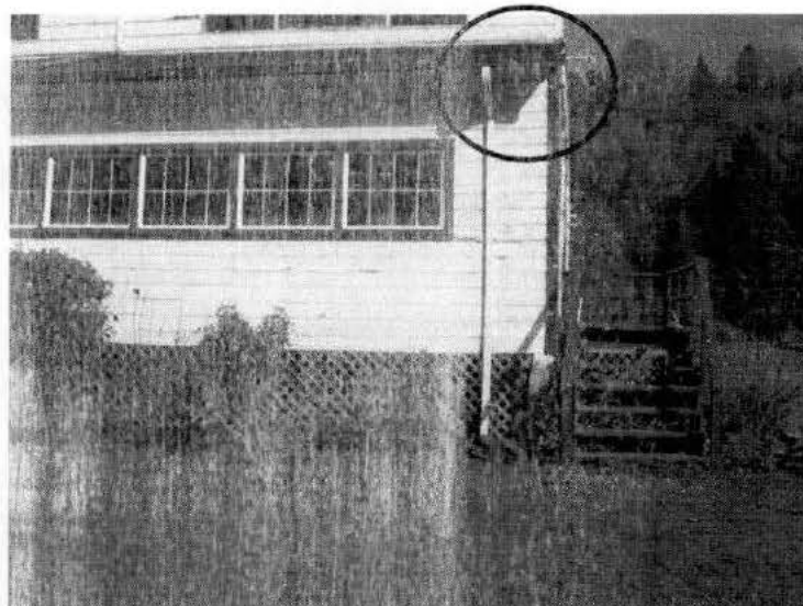
Figure 4.13: Southeast corner of arena – downspout and gutter construction problems, February 2005.
