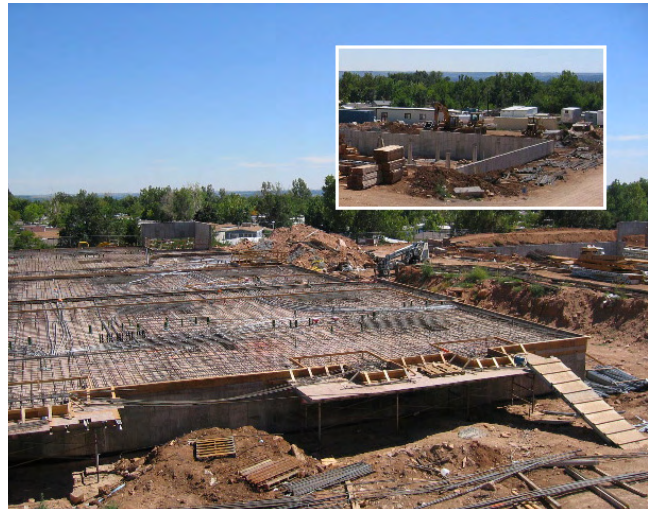
Concrete slab podiums are a more common construction type used for structured parking. Coordination of penetrations is critical.
