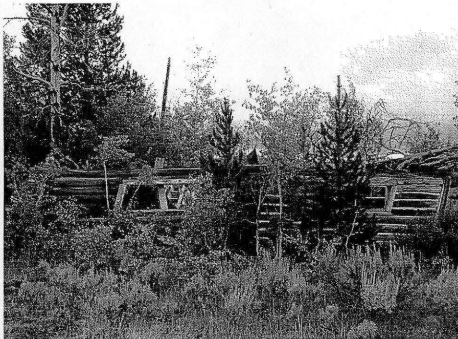
Figure 6.7. Horace Carncross's cabin (HS 1386). 1979 (top) and 2003 (bottom). Many of the structures, like this one, were in poor condition when the park acquired them in 1988. (Top, HABS; bottom, courtesy of Grand Teton National Park)
