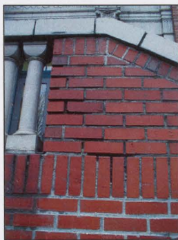
FIGURE 23: MORTAR DISINTEGRATION AT STAIR
