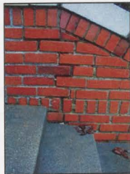
FIGURE 64: MOVEMENT DUE TO JACKING OF THE CORRODED LINTEL
