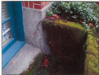
FIGURE 65: CRACKING OF THE STUCCO FINISH ON THE CONCRETE WINDOW WELL RETAINING WALLS
