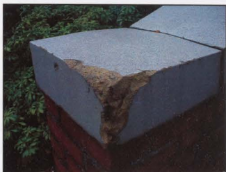
FIGURE 25: SPALLED TERRA COTTA COPING AT STAIR
