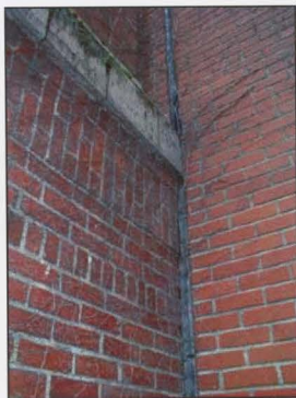
FIGURE 58: DETAIL OF THE EXPANSION JOINT SEAM BETWEEN COMMERCE HALL AND THE 1951 ADDITION
