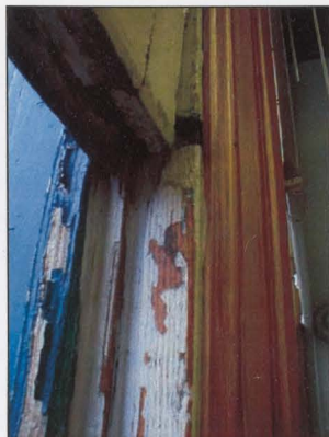
FIGURE 37: PAINT DETERIORATION AND DESICCATION OF WINDOW JAMB AND SASH.
