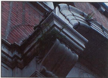
FIGURE 29: VEGETATION TAKING ROOT WHERE THE MORTAR HAS DISINTEGRATED DUE TO WATER INFILTRATION
