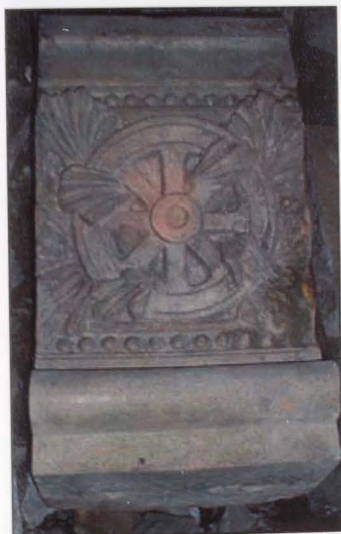
FIGURE 103: PILASTER CAPITAL Type: Pilaster capital Number: 1 each Glazing: Glazed buff clay body Size: 27"x15 1/2" x 14" Condition: Good condition Original Location: Extra piece
