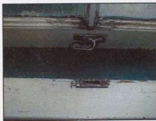
FIGURE 74: WINDOW HARDWARE AND DAMAGE AT MULLION
