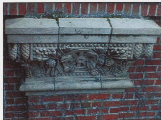
FIGURE 70: MOSS GROWTH ON THE MORTAR JOINTS BETWEEN THE TERRA COTTA PIECES AND VINES ON THE BRICKS IN THE LOWER FLOORS
