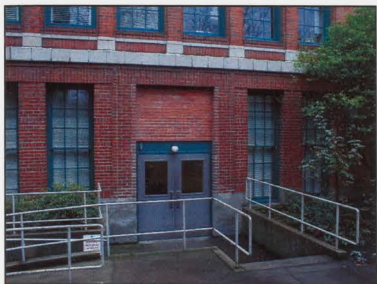
FIGURE 14: HANDICAP RAMP AT EAST ENTRY, 1975 NOTE THAT THE TRANSOM WAS BRICKED-IN
