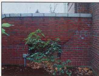
FIGURE 24: CORRODING LINTEL LIFTING STAIR WALL
