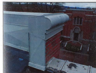
FIGURE 69: SHEET METAL FLASHING WHERE THE CAVITY WALL AND GABLED PARAPET WAS REMOVED
