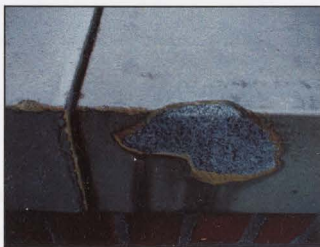
FIGURE 26: GROUT PATCH OF SPALLED TERRA COTTA. NOTE THE MORTAR DISINTERGRATION BETWEEN THE COPING PIECES.
