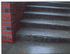
FIGURE 62: DAMAGED CONCRETE NOSING
