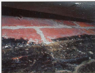
FIGURE 28: A MOIST ENVIRONMENT IS NOT APPARENT BEHIND THE PROTECTION OF THE COPPER FLASHING ON THE PARAPET WALL
