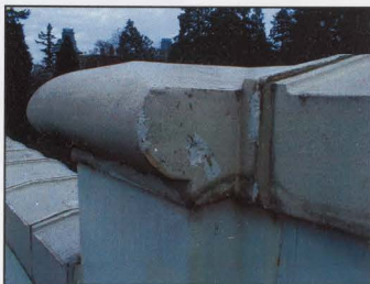
FIGURE 31: SOME IN-PAINTED REPAIR WORK IS PEELING ON PARAPET
