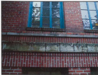
FIGURE 66: STAINING AND ORGANIC DEBRIS ON THE BELT COURSES AND WINDOWS SILLS
