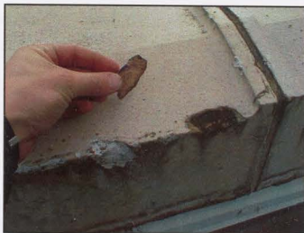
FIGURE 30: SPALLED TERRA COTTA COPING ON PARAPET
