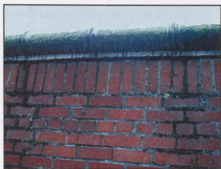
FIGURE 68: STAINING AND GROWTH ON THE DRIP EDGE OF THE TERRA COTTA PARAPET COPING. HEAVY BUILD-UP ON THE MORTAR JOINTS BELOW
