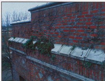
FIGURE 27: ACCUMULATION OF MOSS AND VEGETATION ON THE ENTABLATURE ABOVE THE THIRD FLOOR
