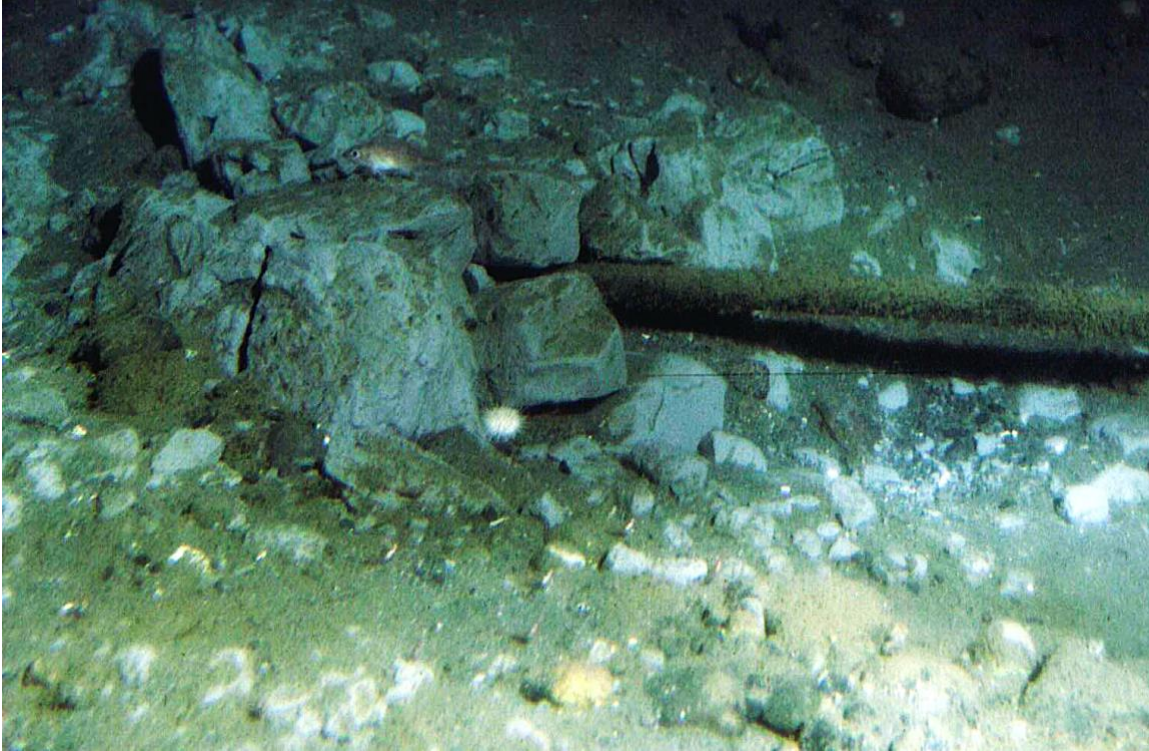
Figure 5.3. A section of the PC-1 cable is buried under rocks and suspended above the seafloor. Suspensions are dangerous for fishing nets and passing marine life. Image courtesy of Olympic Coast National Marine Sanctuary, National Oceanographic and Atmospheric Association, Port Angeles, Washington.
