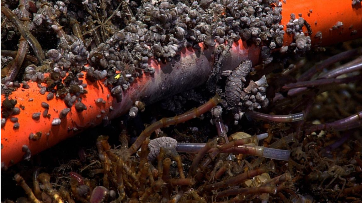
Figure 4.3. Tubeworms, sea spiders, scale worms, limpets, and gastropods colonize and use a deep-sea cable. Early cable designers feared that marine life would infiltrate a cable's exterior. Image courtesy of Ocean Networks Canada/CSSF-ROPOS.
