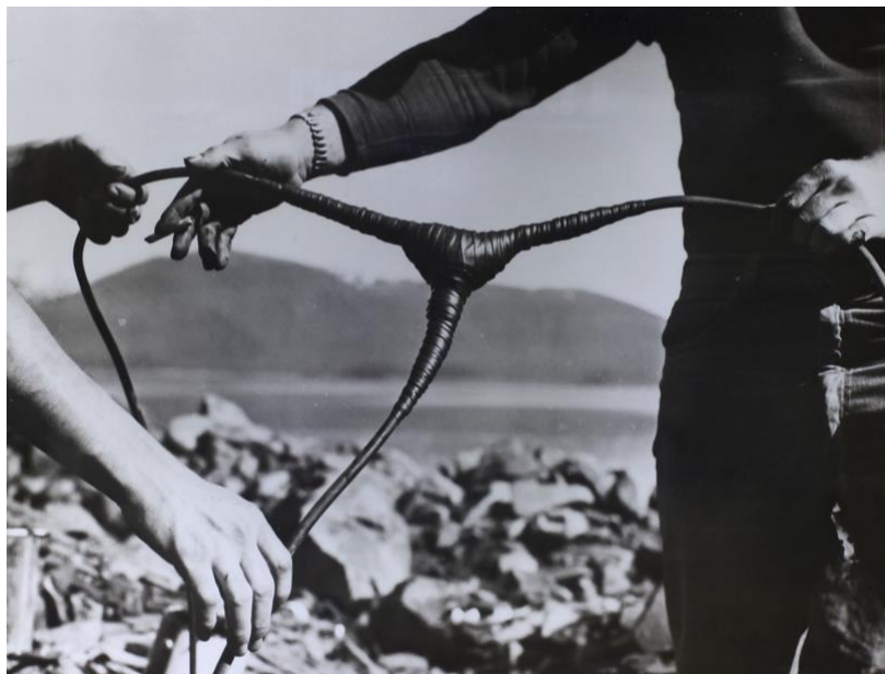
Figure 4.5. Two workers splice a cable at Sokolof Island in southeastern Alaska, ca. 1940s. MS 11-11-7-5, Alaska Communications System Manuscript Collection, Alaska State Library, Juneau.
