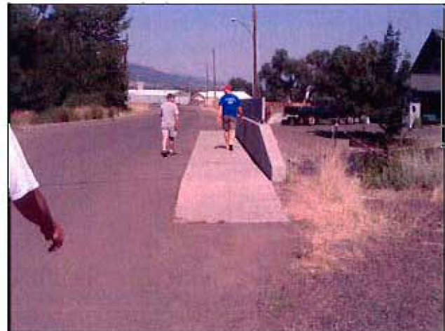
A short sidewalk segment exists on the W McCully Avenue bridge over Wrenn Dobbin Ditch.
