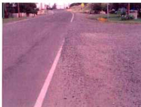
Figure 2-12: Gravel on the E Wallowa Avenue roadway shoulder creates difficult bicycling conditions.
