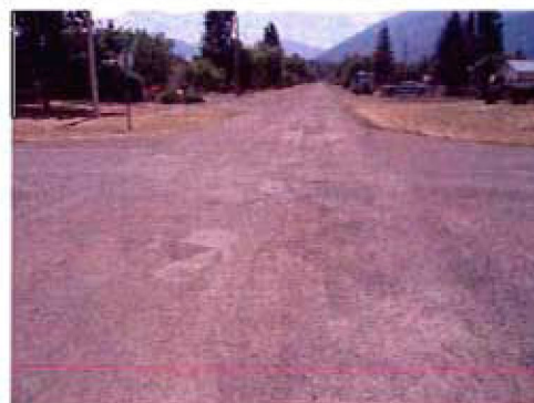
Figure 2-11: Bicyclists encounter marginal/poor pavement conditions on segments of College Street.
