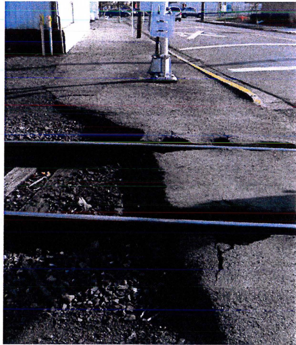
Substandard pedestrian crossing, Douglas Avenue
