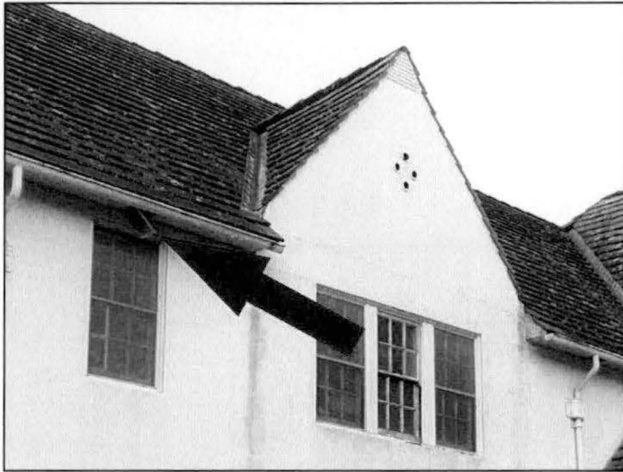
Photograph A.84. Vent screen is detaching from the vent in the eave.
