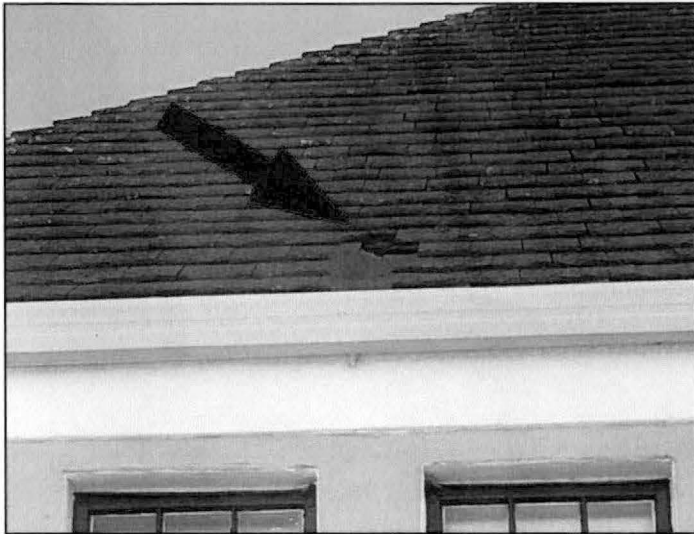
Photograph A.97. Several slate roof tiles missing.
