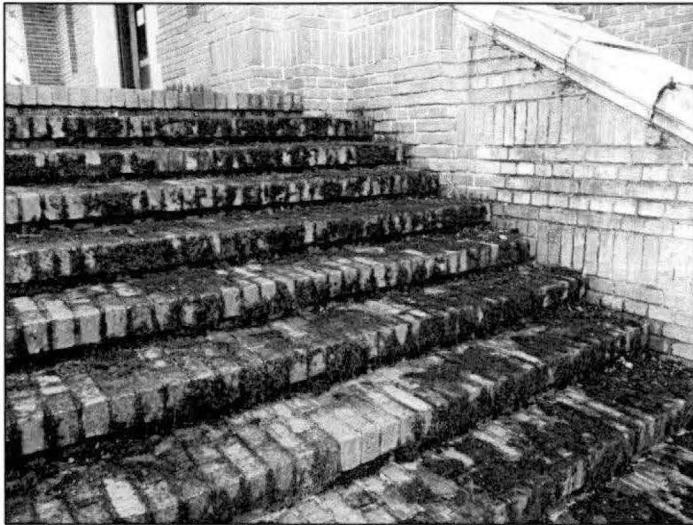
Photograph A.114. Biological growth on brick stairs.
