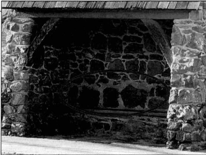
Photograph A.32. Inappropriate repointing on interior wall.
