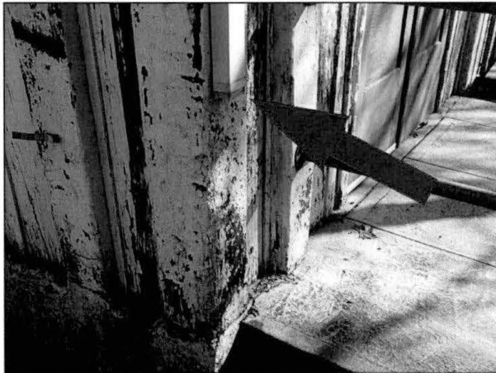
Photograph A.25. Broken downspout.
