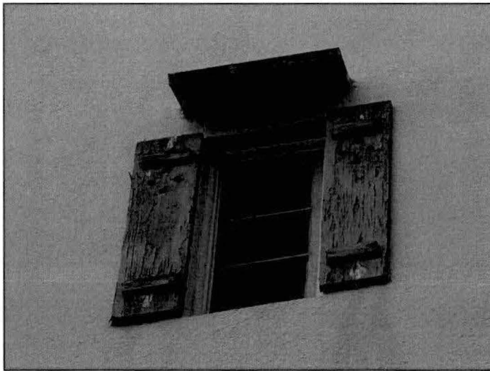
Photograph A.83. Minor paint peeling on decorative window shutters.
