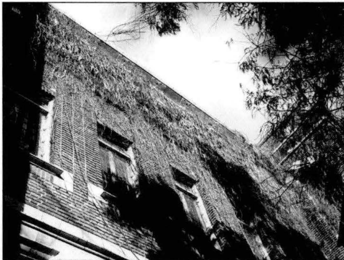
Photograph A.115. Severe climbing vegetation at the eaves on the north elevation.
