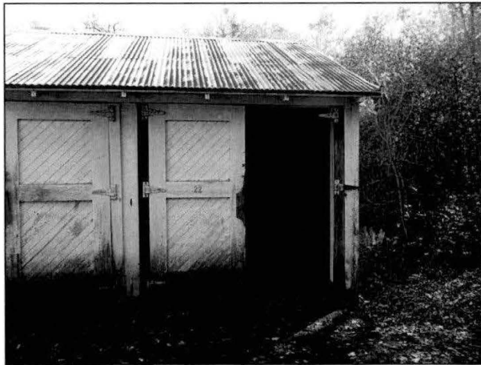
Photograph A.16. Missing garage door on upper level.
