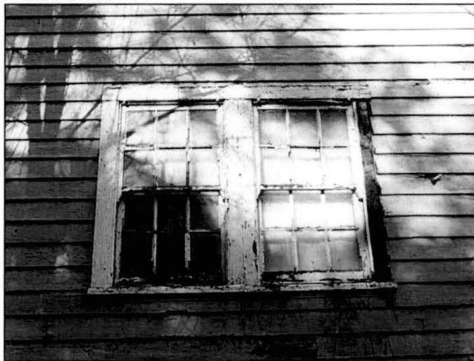
Photograph A.232. Severe paint chipping of wood windows and wood window casings.
