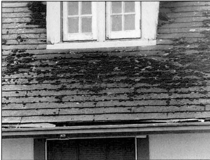
Photograph A.142. Moderate biological growth on composition shingle roofing.
