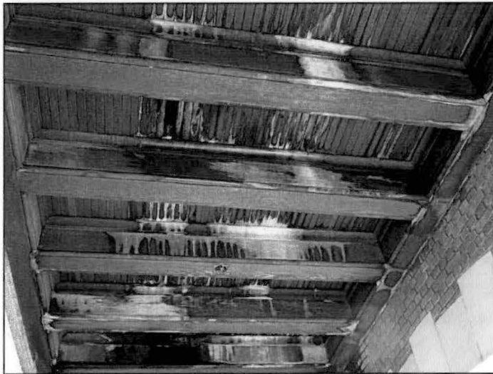
Photograph A.112. Severe moisture infiltration of wood sheathing in projecting entry porch.
