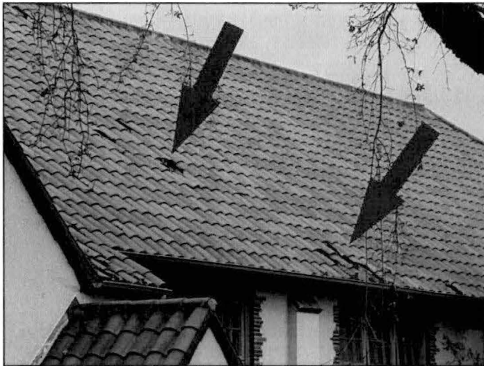
Photograph A.74. Minor roofing damage: broken tiles.
