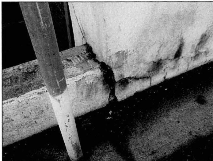
Photograph A.21. Severe cracking of concrete sill wall.
