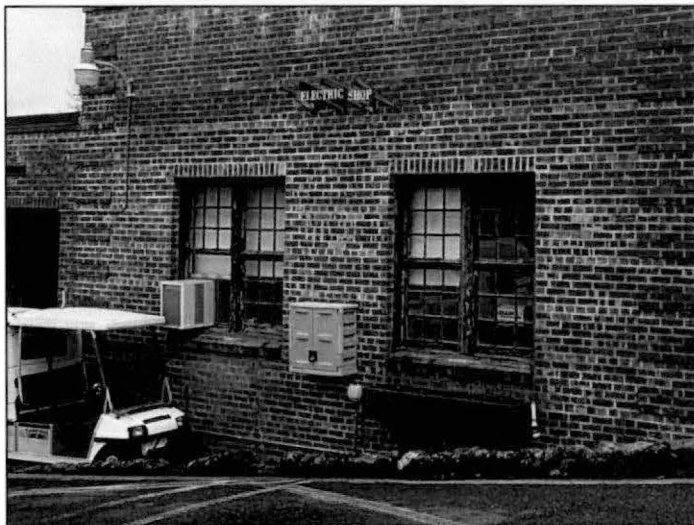
Photograph A.127. Inappropriate repointing of the brick surrounding the windows.
