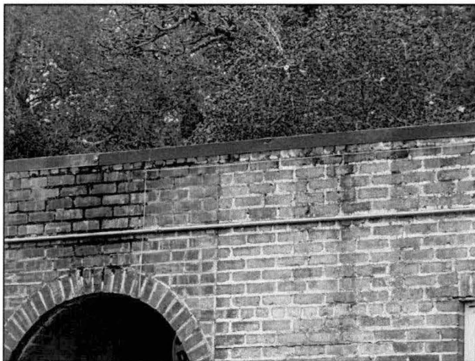
Photograph A.154. Severe efflorescence on brick exterior.
