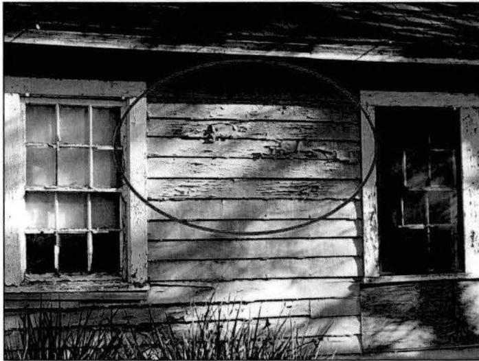
Photograph A.233. Severe deterioration of wood siding.
