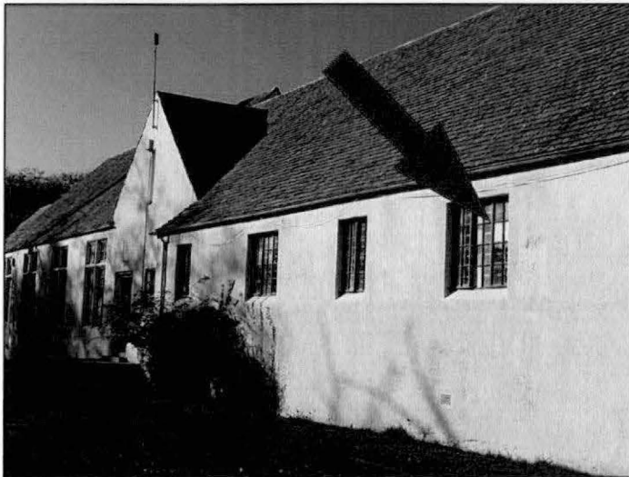
Photograph A.70. Broken window glazing replaced with opaque material.
