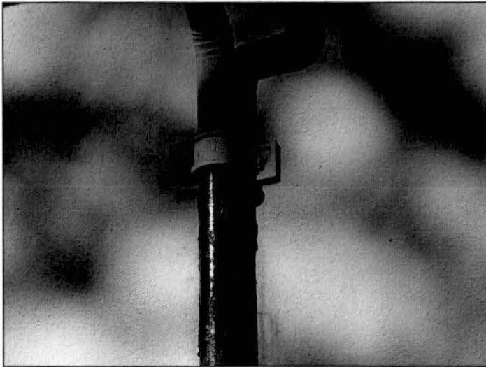
Photograph A.82. Corroding and leaking downspout.
