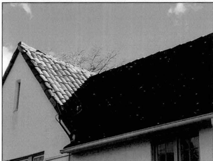
Photograph A.163. Minor biological growth on ceramic tile roofing.
