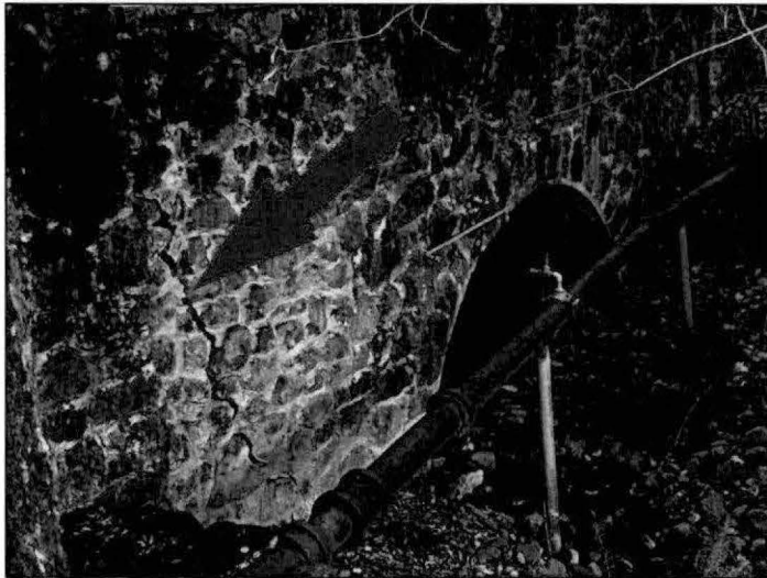
Photograph A.217. Severe cracking of stone masonry.
