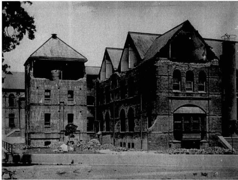
Photograph 2.2. 1906 photograph of earthquake damage.
