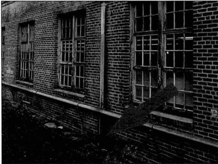
Photograph A.130. Corroding and broken downspout.
