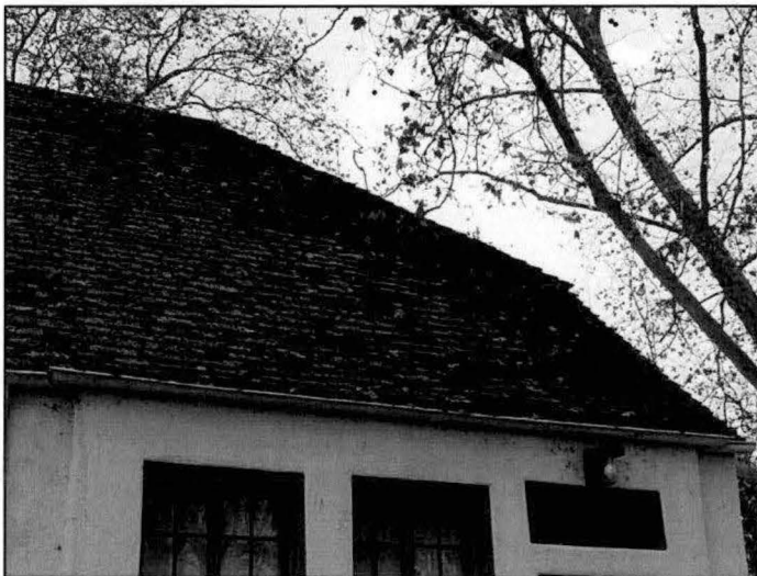
Photograph A.90. Moderate biological growth on roof tiles.
