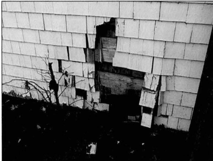
Photograph A.212. Severe deterioration of wood siding, exposing the structure's wood frame.
