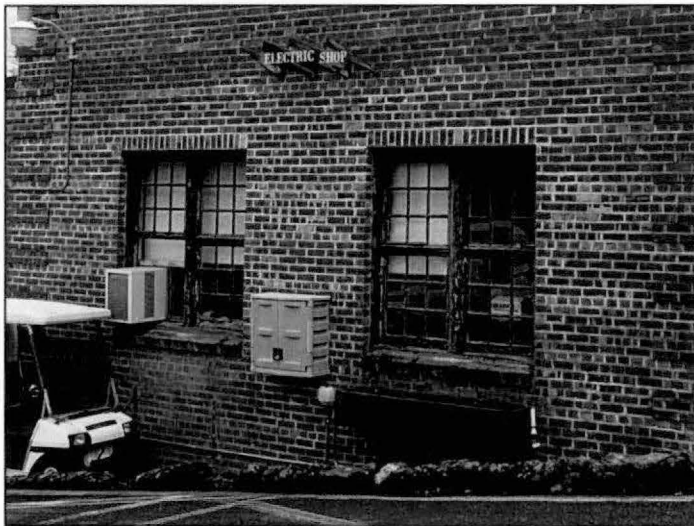
Photograph A.129. Severe paint peeling on wood windows
