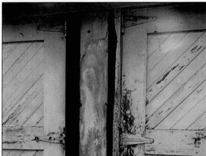
Photograph A.17. Gaps in exterior envelope, caused by broken wood siding between the garage doors.
