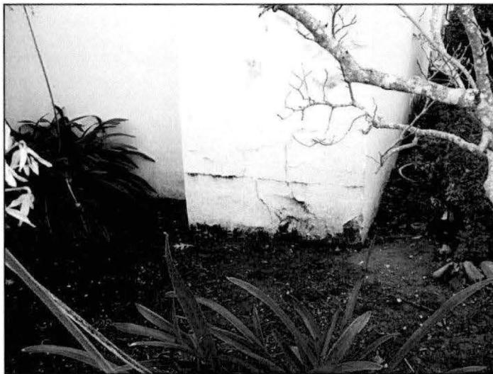
Photograph A.162. Minor rising damp on stucco exterior.
