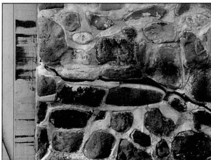
Photograph A.178. Severe cracking in stone.
