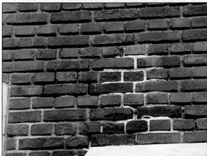
Photograph A.108. Inappropriate repointing.
