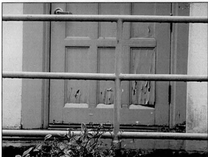
Photograph A.191. Moderate paint peeling on main entry door.
