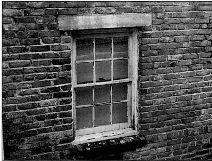
Photograph A.158. Paint chipping on wood windows.
