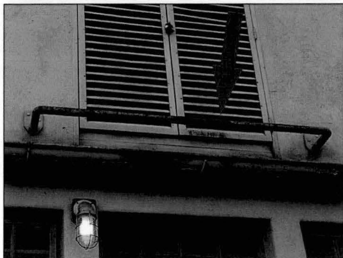
Photograph A.169. Severe corrosion of metal railing.
