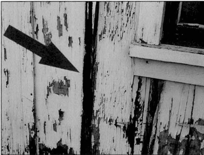
Photograph A.27. Missing wood battens.
