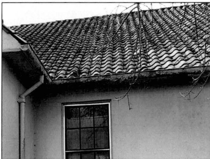
Photograph A.43. Corroding gutters.
