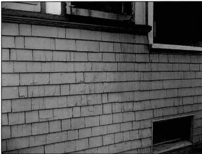
Photograph A.204. Moderate moisture infiltration on wood shingle siding.
