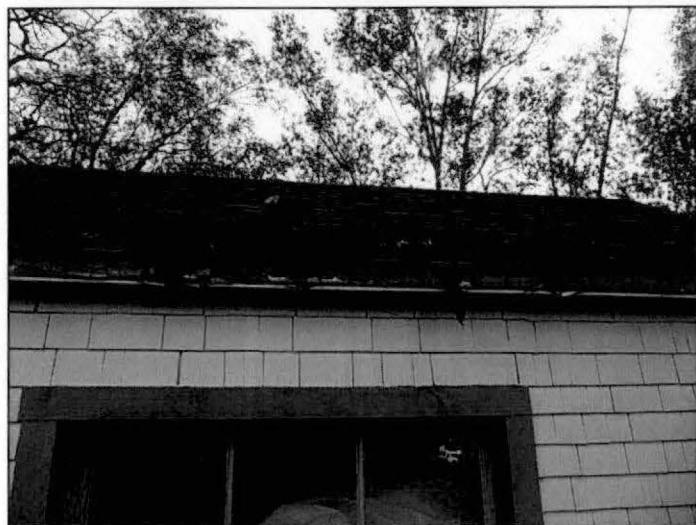
Photograph A.213. Severe biological growth on composition shingle roofing.
