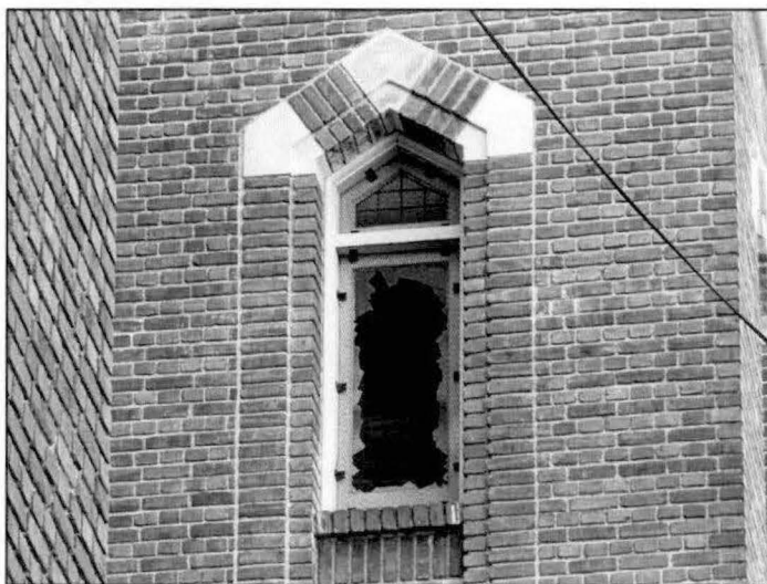
Photograph A.117. Several windows have broken glazing.
