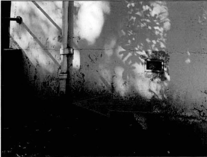
Photograph A.54. Broken downspout.
