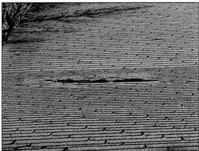
Photograph A.23. Severe deterioration of composition shingle roofing.
