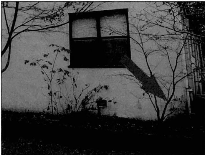
Photograph A.190. Minor rising damp on stucco.
