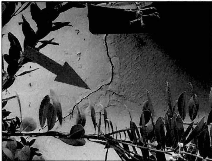
Photograph A.59. Moderate cracking of concrete.
