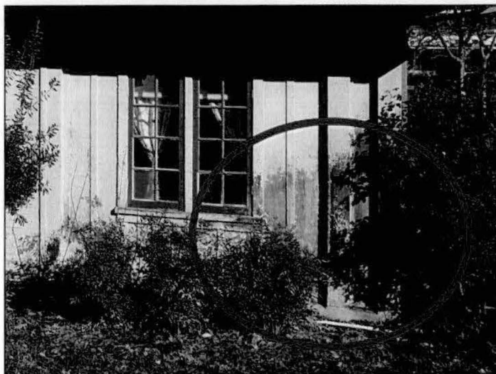
Photograph A.22. Moderate rising damp on wood siding.
