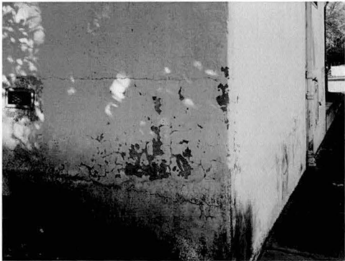
Photograph A.55. Chipping of exterior paint on concrete.
