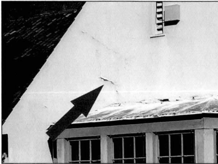
Photograph A.241. Minor paint chipping on stucco exterior.
