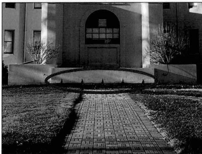
Photograph A.38. Minor moisture infiltration on sill wall due to five drain openings allowing water to drain onto the stucco.
