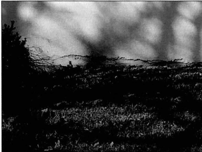
Photograph A.228. Minor chipping of stucco near soil level.
