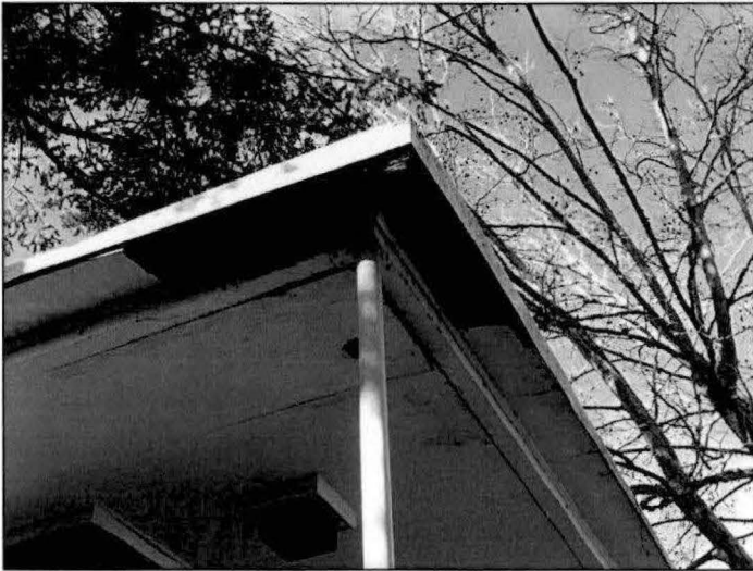
Photograph A.91. Broken soffit boards on porch overhang.
