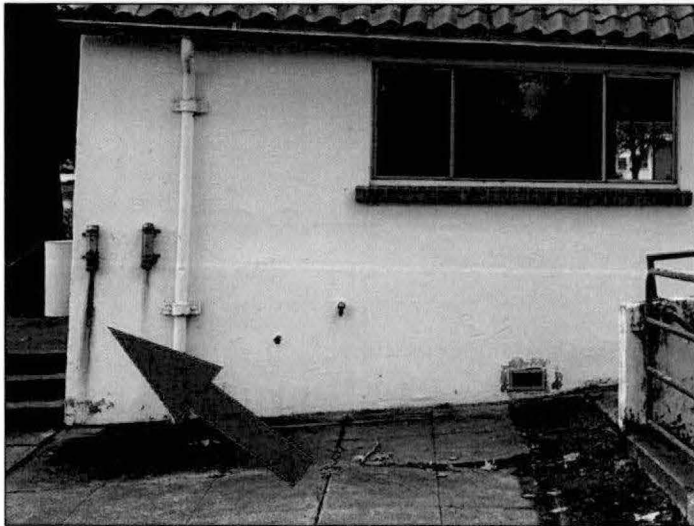
Photograph A.52. Rust staining on concrete from corroding exterior metal components.
