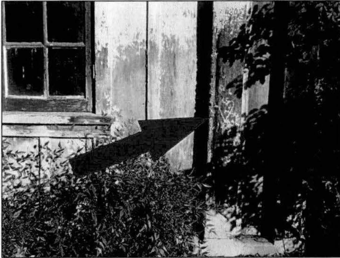
Photograph A.26. Vandalism in the form of carvings in the wood siding.
