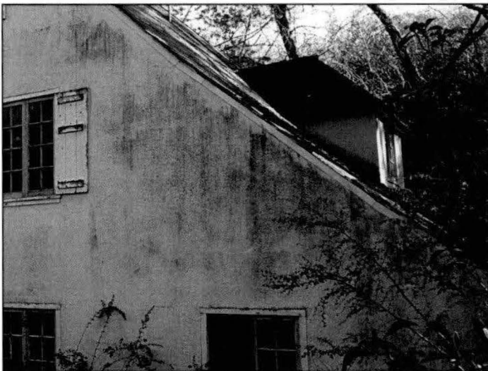
Photograph A.4. Severe moisture infiltration on exterior stucco.
