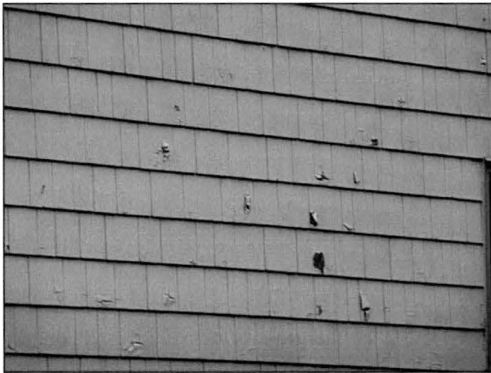
Photograph A.185. Minor paint peeling on wood shingles.
