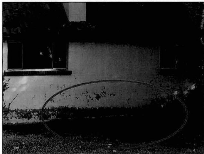
Photograph A.51. Severe rising damp on concrete.
