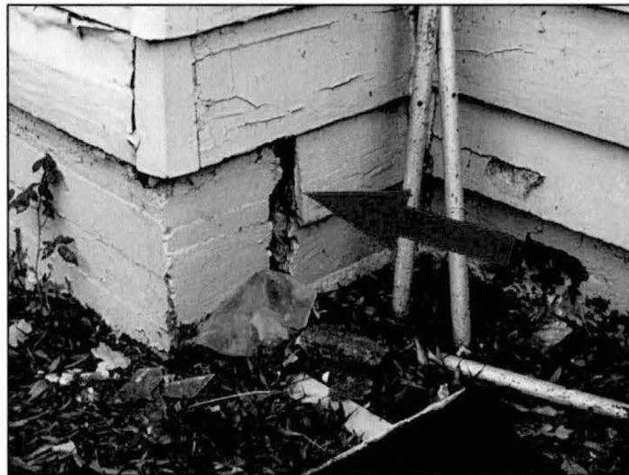
Photograph A.234. Severe cracking in concrete foundation.
