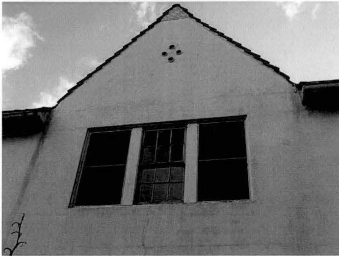
Photograph A.80. Moderate moisture infiltration of stucco.
