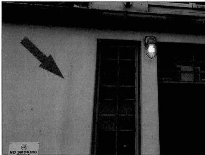
Photograph A.168. Moderate moisture infiltration caused by corroding and leaking gutter.
