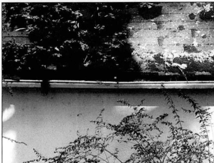
Photograph A.5. Severe biological growth on composite shingle roofing.
