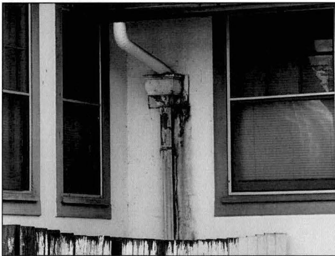
Photograph A.143. Corroding and leaking downspout.
