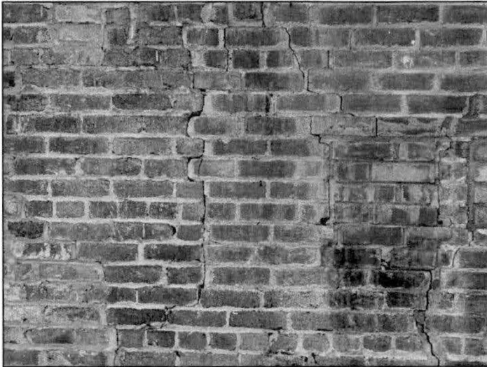
Photograph A.155. Severe cracking in brick wall, through both bricks and mortar.
