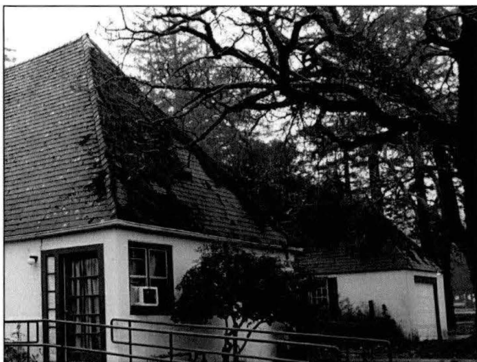
Photograph A.200. Severe biological growth on roofing.
