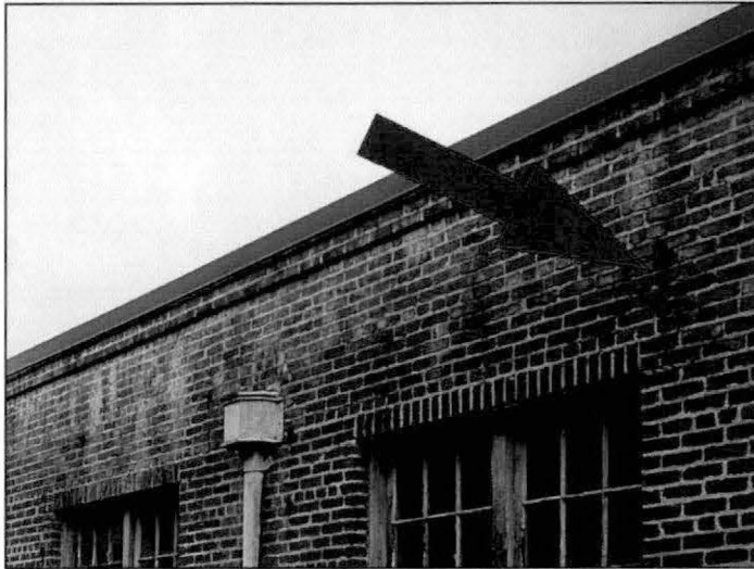
Photograph A.128. Moderate rust staining caused by the corrosion of exterior metal components.
