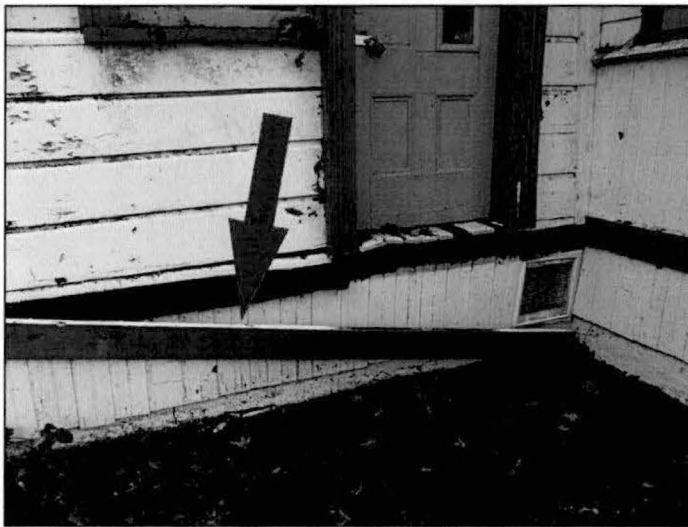
Photograph A.208. Severe siding separation.
