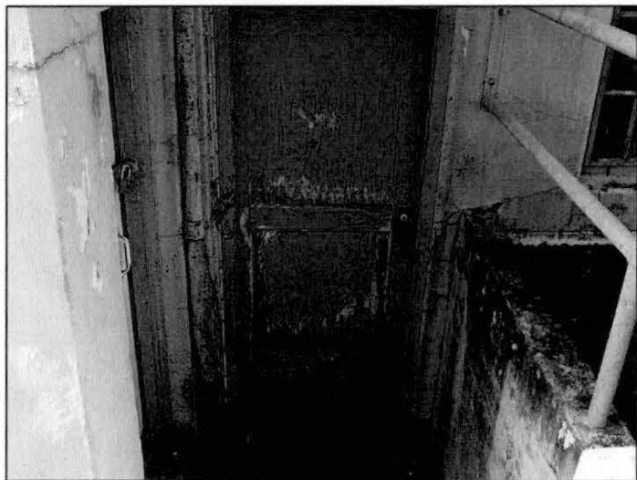
Photograph A.170. Severe corrosion and leaking of the gutter system.
