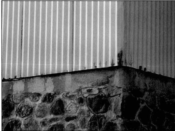
Photograph A.179. Minor corrosion of corrugated metal siding.
