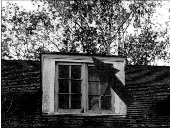
Photograph A.7. Severe corrosion of metal flashing.
