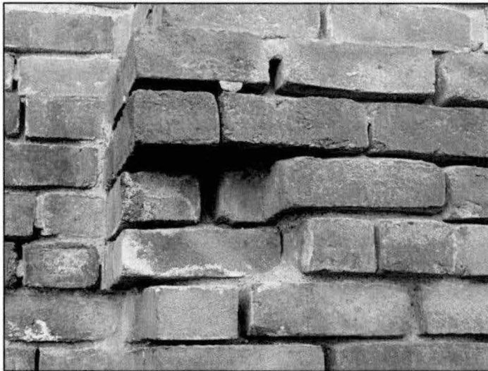
Photograph A.107. Missing bricks.
