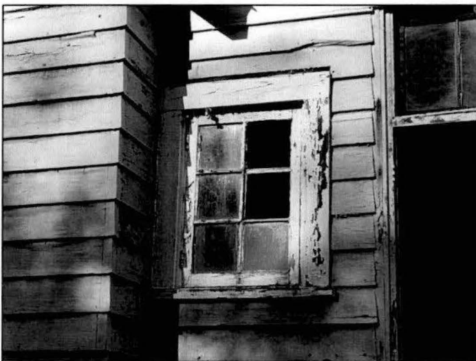
Photograph A.236. Missing window glazings.
