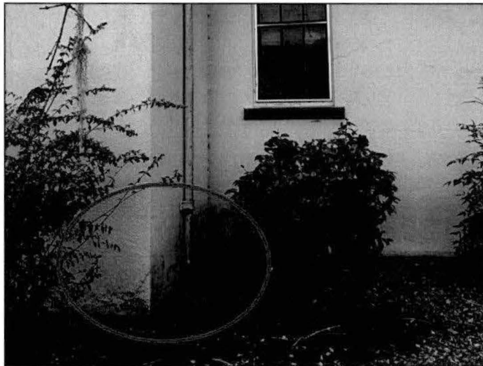
Photograph A.41. Minor rising damp on stucco.
