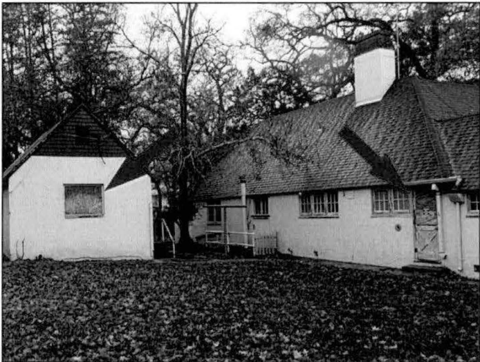
Photograph A.197. A few windows are covered in wood boards.
