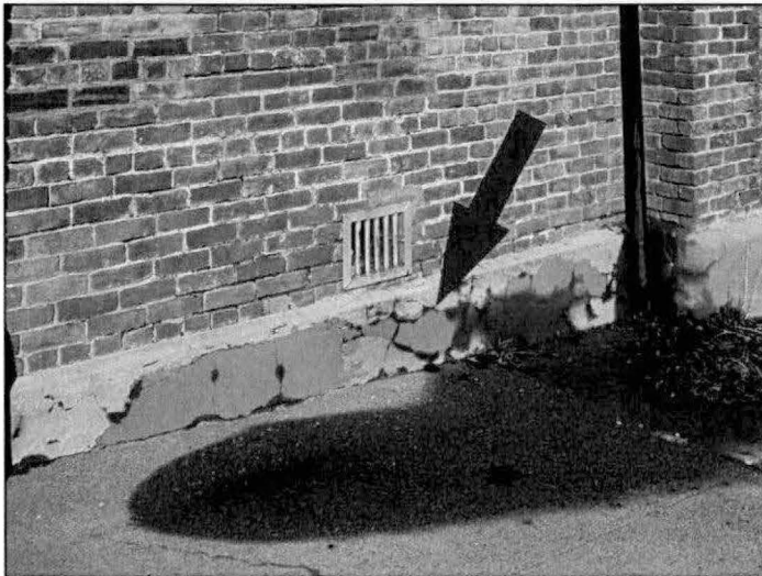
Photograph A.110. Severe hairline cracking on concrete foundation.
