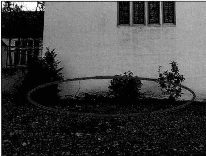
Photograph A.135. Minor rising damp on concrete.
