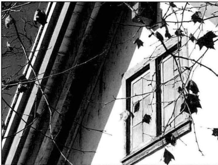
Photograph A.141. Minor rust staining onto concrete from corroding sheathing under eaves.
