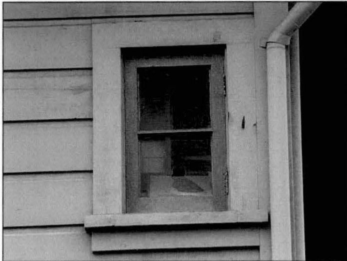
Photograph A.66. Broken window glazing on upper level of northeast elevation.
