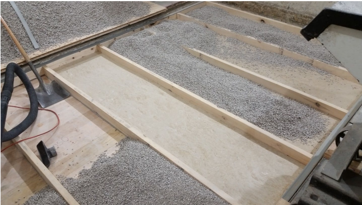
Figure 10 - Hemp boards partially installed between sleepers, gravel partially installed over hemp boards
