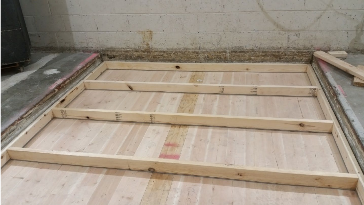
Figure 7 - 2" by 4" sleepers partially installed, with Piano B 40/40 strips fastened to underside of sleepers
