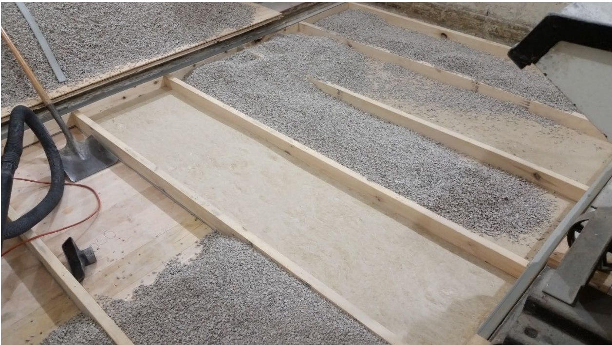
Figure 10 – Hemp boards partially installed between sleepers, gravel partially installed over hemp boards
