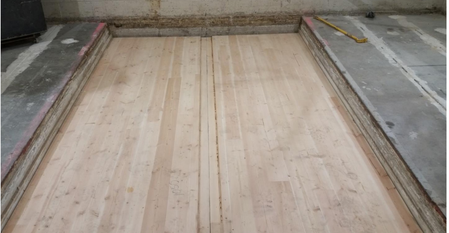
Figure 1 - F03 Assembly - CLT installed in test aperture, with 3/4" x 3" rabbets each along panel-to-panel joint (from above)
