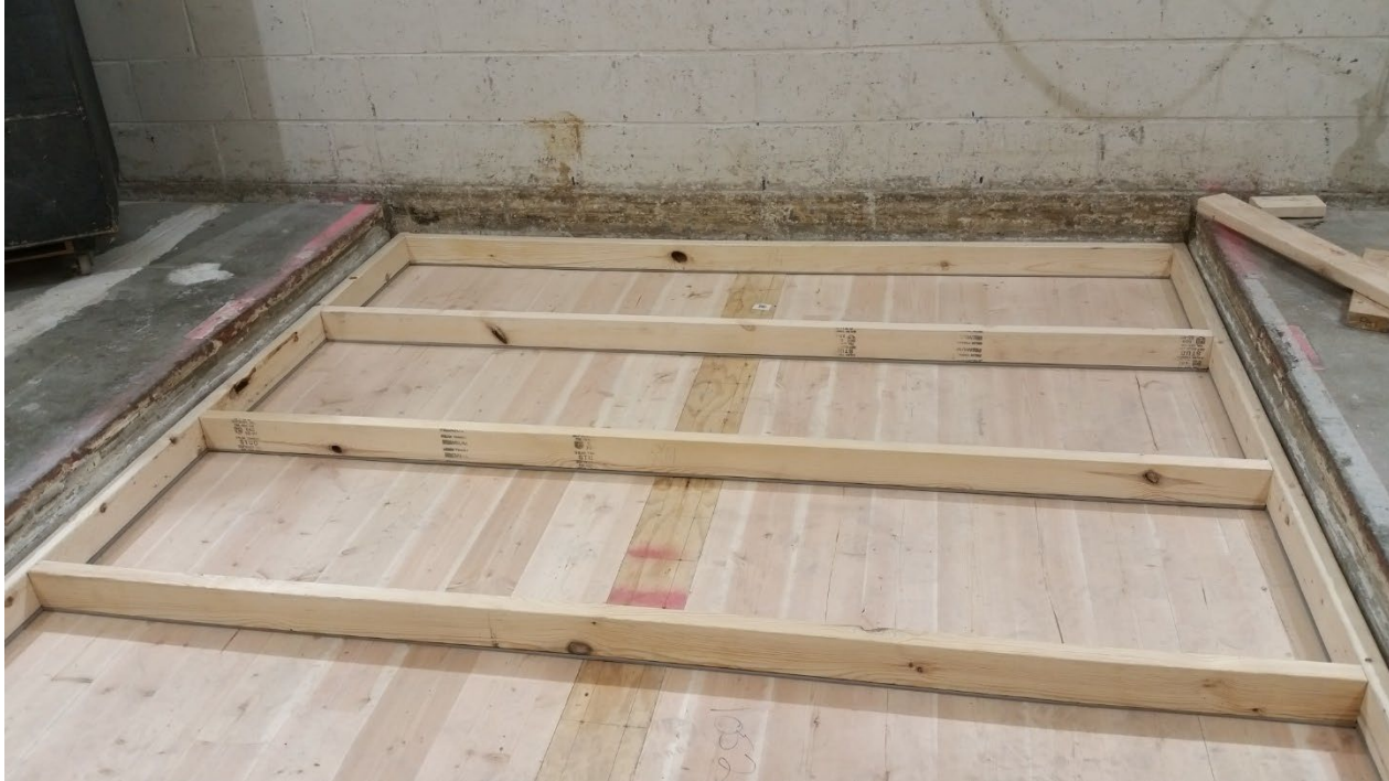
Figure 7 – 2” by 4” sleepers partially installed, with Piano B 40/40 strips fastened to underside of sleepers
