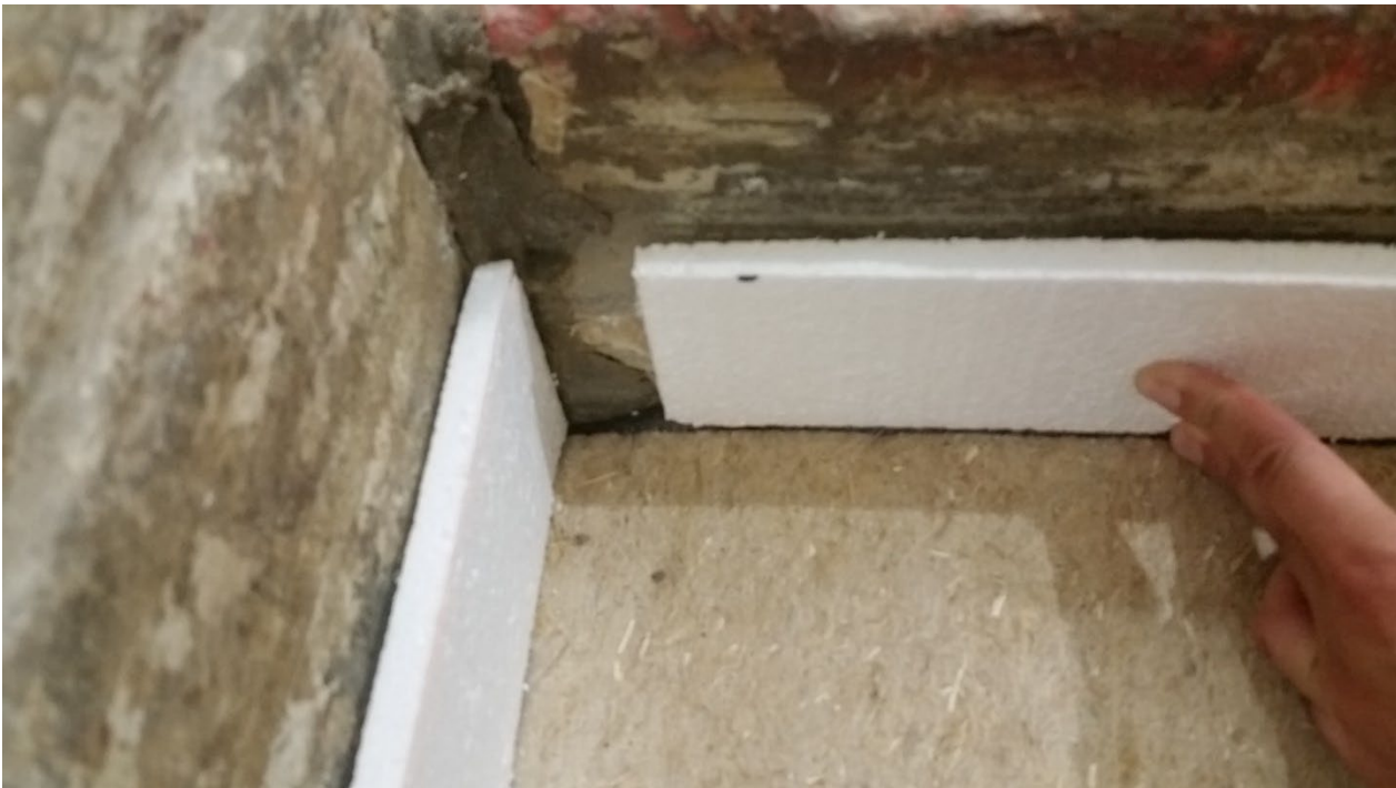
Figure 8 – Polystyrene used as an isolation around the perimeter prior to installation of gravel
