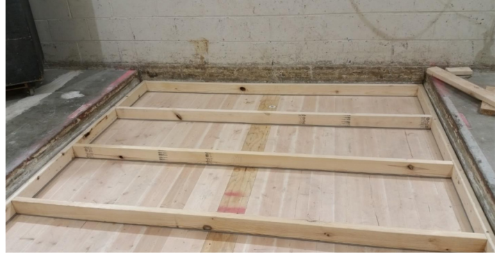
Figure 7 - 2"x4" sleepers partially installed, with Piano B 40/40 fastened to underside of sleepers
