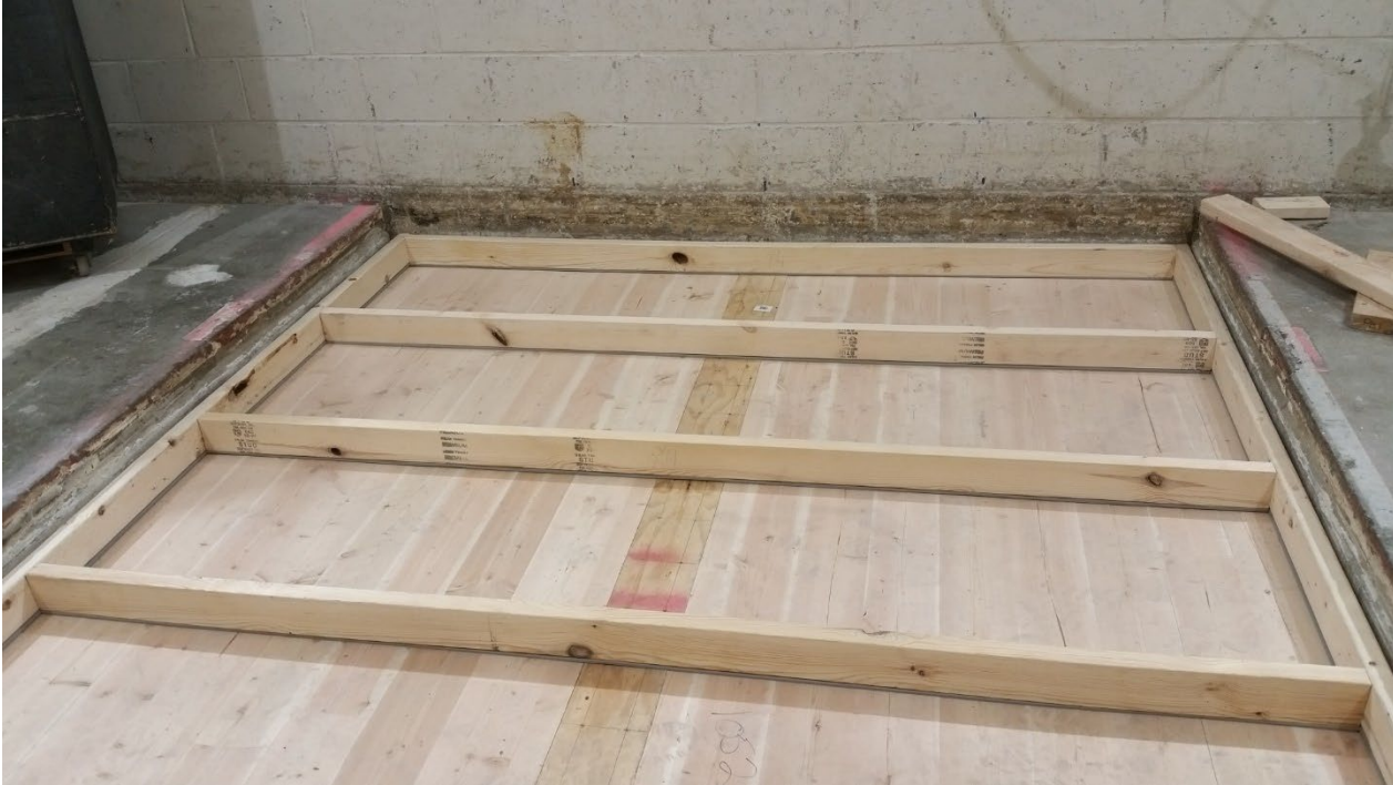
Figure 7 – 2” by 4” sleepers partially installed, with Piano B 40/40 strips fastened to underside of sleepers
