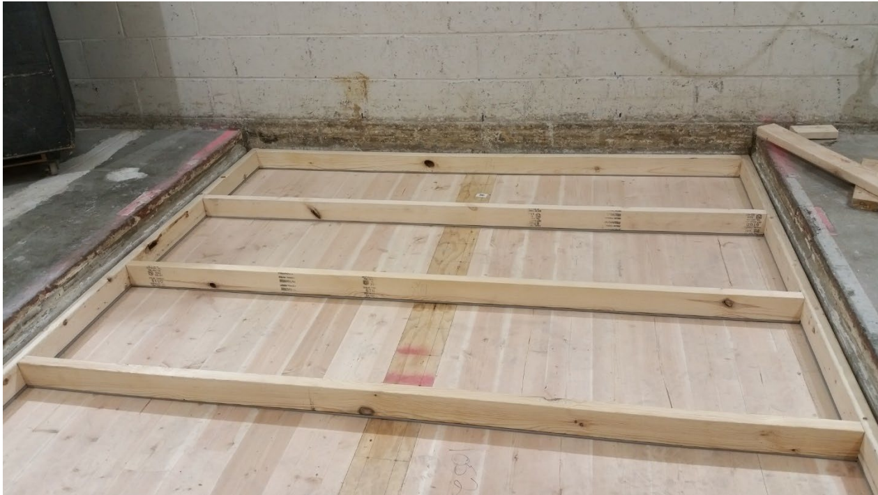
Figure 7 – 2” by 4” sleepers partially installed, with Piano B 40/40 strips fastened to underside of sleepers
