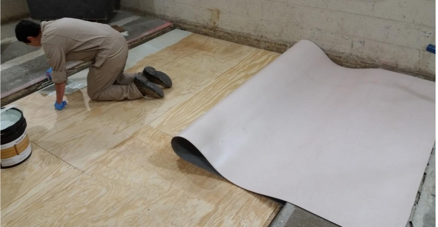
Figure 7 - F03 Assembly - Flooring adhesive, partially installed. Applied before flooring install (from above)
