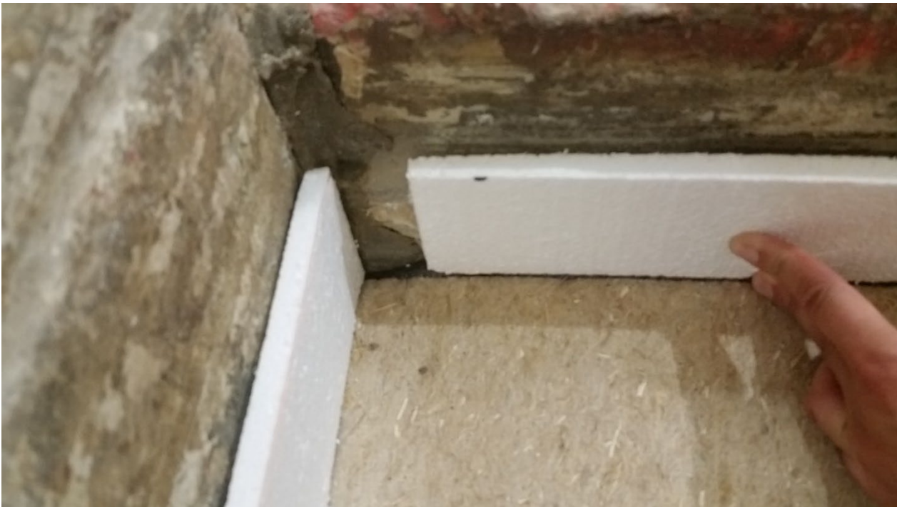
Figure 8 - Polystyrene used as an isolation around the perimeter prior to installation of gravel
