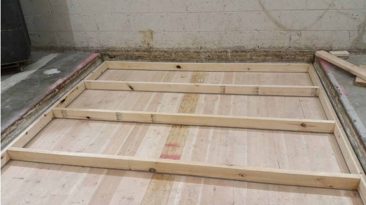
Figure 7 – 2” by 4” sleepers partially installed, with Piano B 40/40 strips fastened to underside of sleepers
