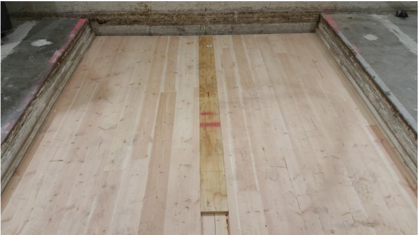
Figure 2 - F03 Assembly - 3/4" x 6" plywood spline partially installed over CLT rabbets (from above)
