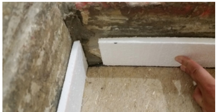
Figure 8 - Polystyrene used as an isolation around the perimeter prior to installation of gravel
