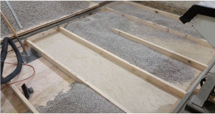
Figure 10 - Hemp boards partially installed between sleepers, gravel partially installed over hemp boards
