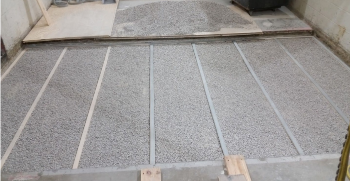
Figure 11 - Hemp boards, gravel, and sleepers installed, Piano B 40/40 strips partially installed over sleepers
