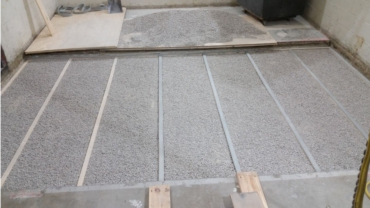
Figure 11 – Hemp boards, gravel, and sleepers installed, Piano B 40/40 strips partially installed over sleepers
