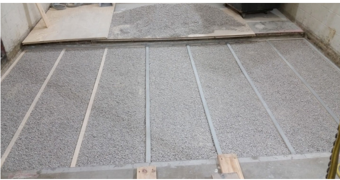
Figure 11 - Hemp boards, gravel, and sleepers installed, Piano B 40/40 strips partially installed over sleepers
