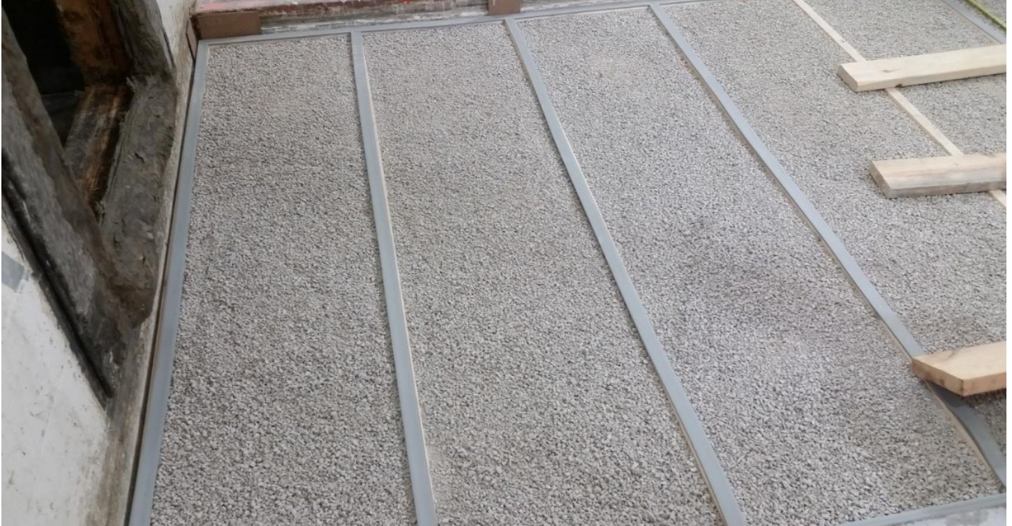
Figure 5 - F03 Assembly - Gravel installed, Piano B 40/40 partially installed on top of sleepers (from above)
