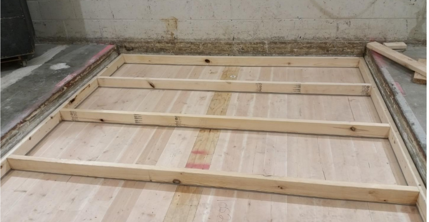
Figure 3 - F03 Assembly - 2x4 sleepers partially installed, with Piano B 40/40 strips fastened to underside of sleepers (from above)
