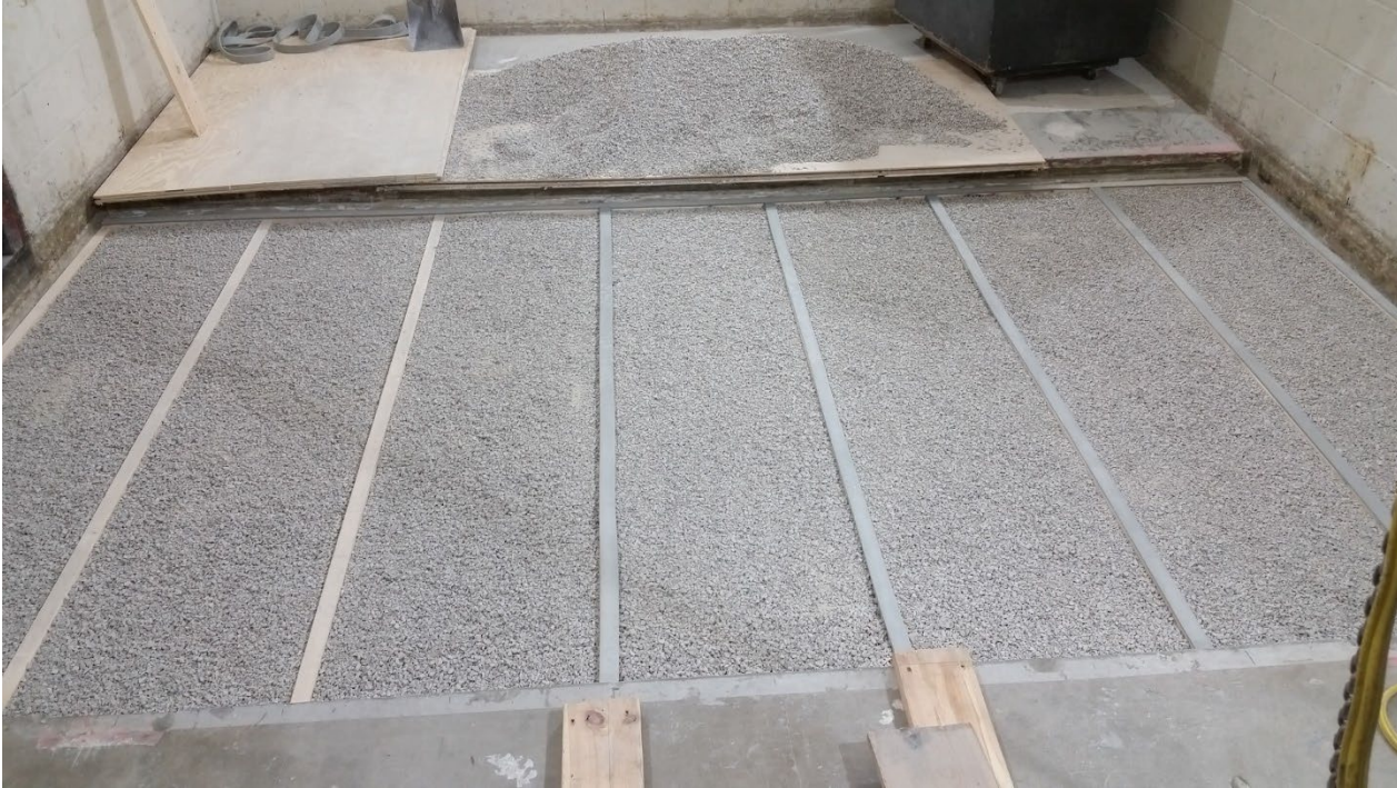
Figure 11 - Hemp boards, gravel, and sleepers installed, Piano B 40/40 strips partially installed over sleepers
