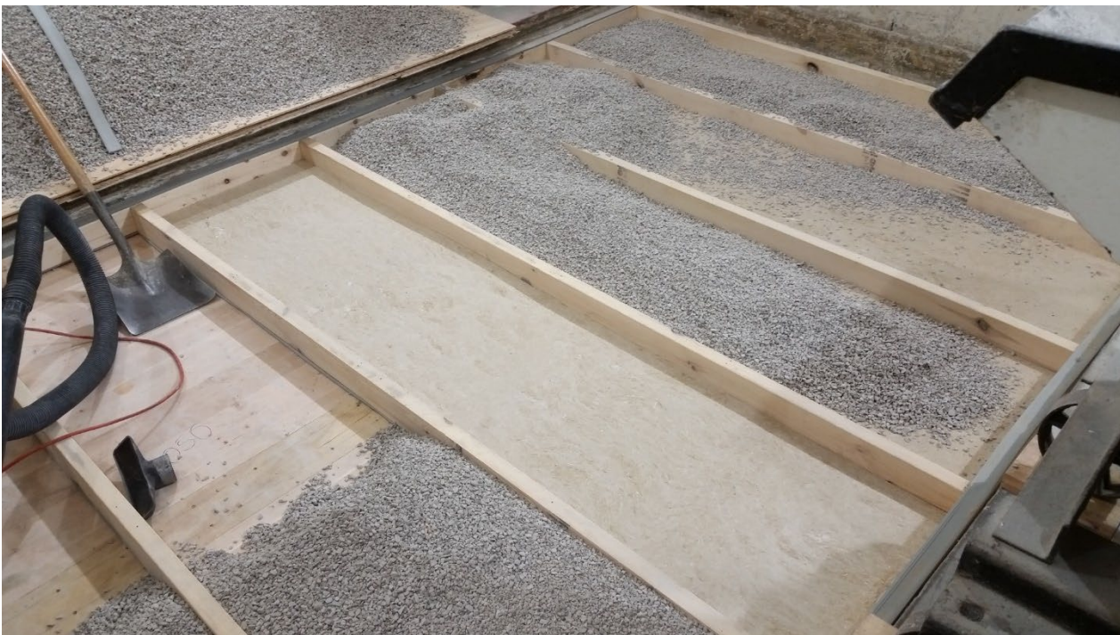
Figure 10 - Hemp boards partially installed between sleepers, gravel partially installed over hemp boards
