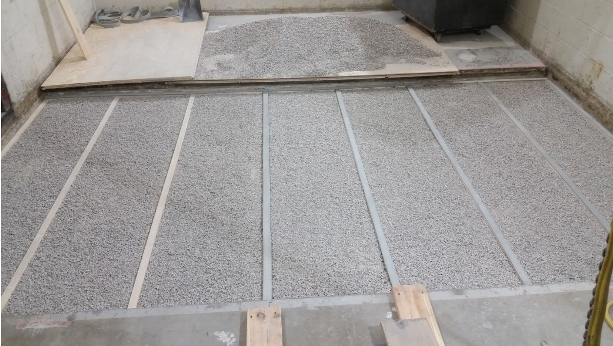
Figure 11 – Hemp boards, gravel, and sleepers installed, Piano B 40/40 strips partially installed over sleepers
