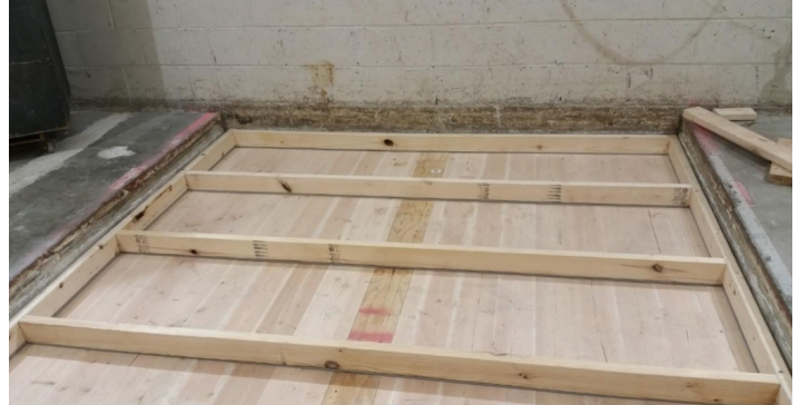
Figure 7 - 2"x4" sleepers partially installed, with Piano B 40/40 fastened to underside of sleepers
