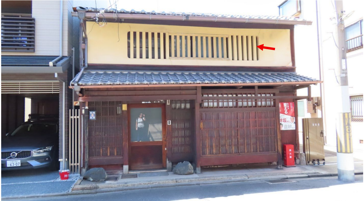
Fig. 2.6 – Upper: Flat-Plastered Style , Lower: Bay-Lattice Style , Kamanza Street, Nakagyō, Kyoto, Red Arrow: mushiko-mado
