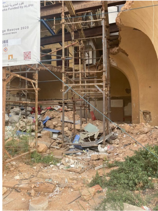
Housing wrecked by the Beirut Blast, still shattered one year after the explosion 6
