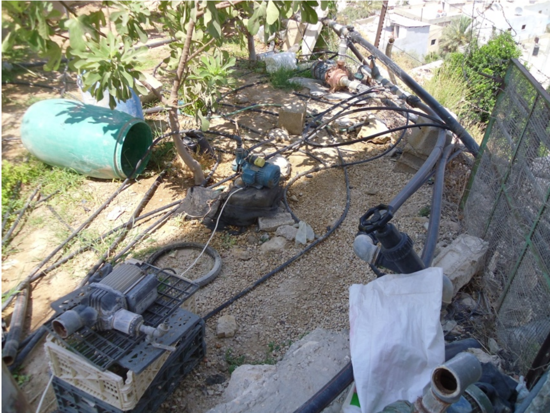
Figure 12: A pressure pump used on Zbeidat's highest elevation, photo by author.
