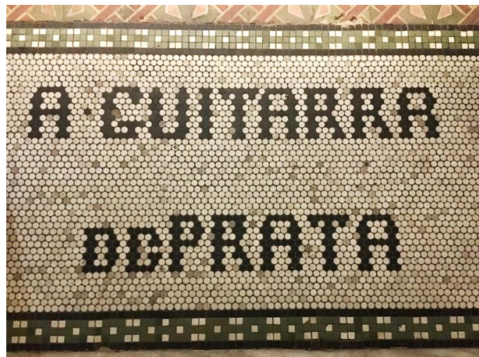
Figure 32 The original tiling for A Guitarra de Prata, the famous instrument store that once functioned in the space that is now the Almerinda Gama House.
