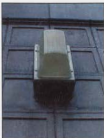
FIGURE 15: HIGH PRESSURE SODIUM LIGHTS REPLACED THE ORNAMENTAL LANTERNS THAT FLANKED THE ENTRY
