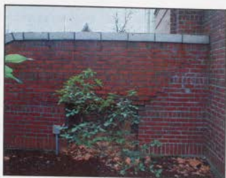
FIGURE 24: CORRODING LINTEL LIFTING STAIR WALL.
