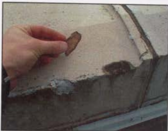
FIGURE 30: SPALLED TERRA COTTA COPING ON PARAPET
