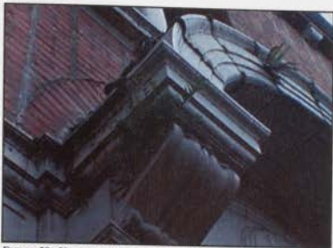
FIGURE 29: VEGETATION TAKING ROOT WHERE THE MORTAR HAS DISINTEGRATED DUE TO WATER INFILTRATION
