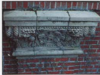
FIGURE 70: MOSS GROWTH ON THE MORTAR JOINTS BETWEEN THE TERRA COTTA PIECES AND VINES ON THE BRICKS IN THE LOWER FLOORS
