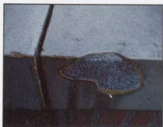
FIGURE 26: GROUT PATCH OF SPALLED TERRA COTTA. NOTE THE MORTAR DISINTEGRATION BETWEEN THE COPING PIECES.
