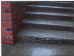
FIGURE 62: DAMAGED CONCRETE NOSING
