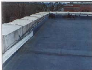
FIGURE 71: FULLY ADHERED ELASTIC ROOF MEMBRANE AFFIXED WITH METAL RETAINING BARS, ANCHORED TO THE PARAPET COPING
