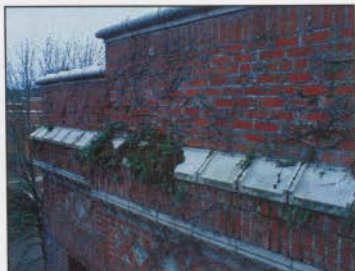
FIGURE 27: ACCUMULATION OF MOSS AND VEGETATION ON THE ENTABLATURE ABOVE THE THIRD FLOOR
