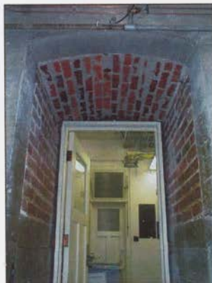
FIGURE 60: SEGMENTAL BRICK ARCH PASSAGE THROUGH THE FOUNDATION WALL TO THE MECHANICAL ROOM
