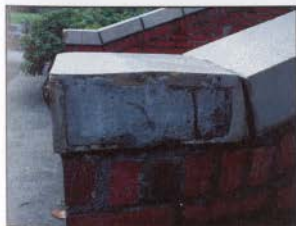
FIGURE 18: ALTERATION OF TERRA COTTA COPING, 1951
