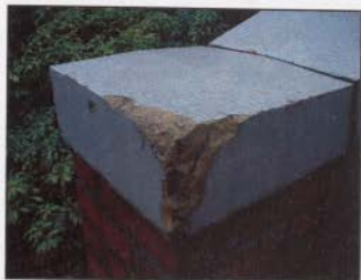
FIGURE 25: SPALLED TERRA COTTA COPING AT STAIR
