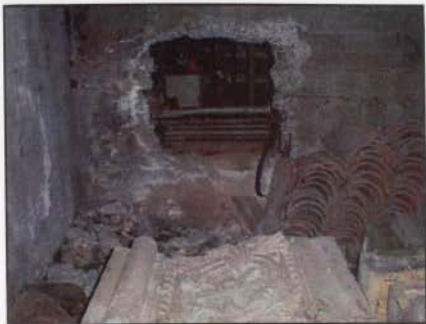
FIGURE 102: STAIR VAULT Hidden access to the stair vault of the Education Building was found off the mechanical room, 112. The terra cotta was found in this space. A pilaster capital and a stack of terra cotta roofing tiles are pictured in the foreground.
