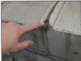
FIGURE 72: LATEX SEALANT BETWEEN PARAPET COPING
