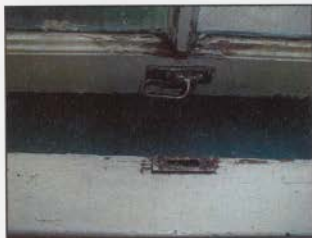
FIGURE 74: WINDOW HARDWARE AND DAMAGE AT MULLION
