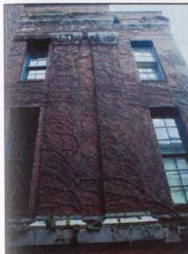
FIGURE 11: PILASTERS AT NORTH ELEVATION. NOTE VINES AND GROWTH.
