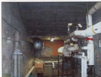
FIGURE 59: FOUNDATION STEM WALL UNDER STAIR VAULT. NOTE THE COLD JOINTS AND THE BOARD FORMED MARKS
