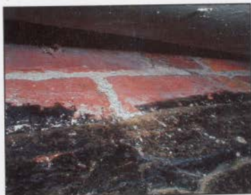
FIGURE 28: A MOIST ENVIRONMENT IS NOT APPARENT BEHIND THE PROTECTION OF THE COPPER FLASHING ON THE PARAPET WALL
