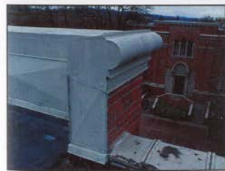
FIGURE 69: SHEET METAL FLASHING WHERE THE CAVITY WALL AND GABLED PARAPET WAS REMOVED
