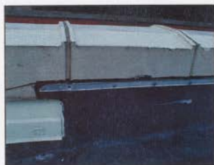
FIGURE 33: LEAD ANCHOR NAILS INSTALLED THROUGH TERRA COTTA COPING TO HOLD THE ROOF MEMBRANE'S RETAINING BAR
