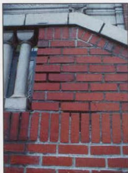
FIGURE 23: MORTAR DISINTEGRATION AT STAIR
