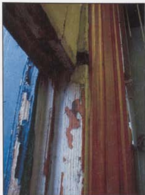
FIGURE 37: PAINT DETERIORATION AND DISICCATION OF WINDOW JAMB AND SASH.
