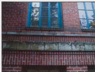
FIGURE 66: STAINING AND ORGANIC DEBRIS ON THE BELT COURSES AND WINDOWS SILLS
