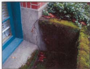
FIGURE 65: CRACKING OF THE STUCCO FINISH ON THE CONCRETE WINDOW WELL RETAINING WALLS
