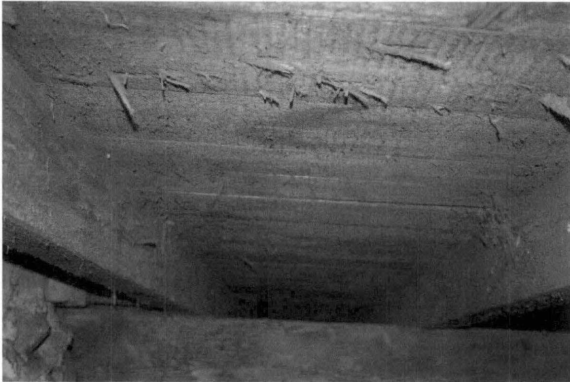
Fig. V-6. Near the top of this photo is evidence of machine cut and wire nails protruding through the first layer of flooring into the crawlspace. Note that they are in line, following butt joints in the second layer of flooring above. It suggests that a wall was likely affixed to the other side of the flooring through toe nailing, and corroborates the evidence in the room above that there was a former division in this room between Rooms 1 and 2 at this location. This example is just west of the restored east hearth under Room 2 (E5). Photograph by Aaron Lemchen March 2005.
