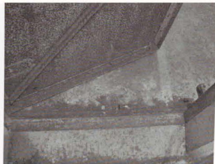
Photo 52. (Above.) Slightly elevated door threshold to raise level of air lock above tunnel. Note traces of red primer visible in these photos.
