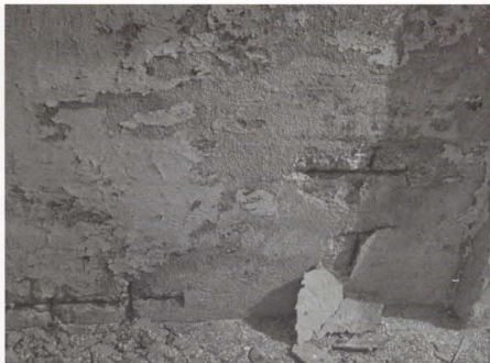
Photo 67. (Left). Peeling paint and spalled concrete with exposed rebar indicate moisture problems in the west wall of the dormitory. The concrete in this section of the casemate was poured directly against the rock outcrop of Chinook Point.
