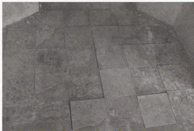
Photo 32. (Above). Closeup of doorway showing spalls with exposed rebar and cracking with stalactites.
