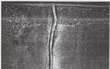
Figure 19. A high-speed grinder is used to widen a crack in preparation for installation of a sealant. This process is called "routing." After the crack is prepared, the sealant is installed to prevent moisture infiltration through the crack. Although sealant repairs can provide a durable, watertight repair for moving cracks, they tend to be very visible.
