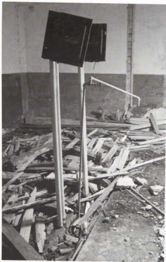
Photo 77. (Above). Two electrical control boxes in what would have been the engine room of the casemate.
