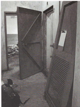
Photo 51. (Above.) Non gas-proof door to battery room has been removed and is currently in tunnel outside east air lock.
