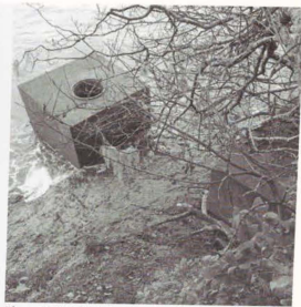
Photo 89. Manhole leading to cable tunnel. Local lore says that this is the preferred point of unauthorized entry to the casemate. The lower box is part of the 1944 improvements.
