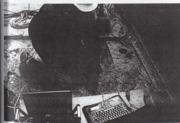
Figure 16. Impact echo testing is performed on a concrete structural slab to help determine depth of deterioration. In this method, a short pulse of energy is introduced into the structure and a transducer mounted on the impacted surface of the structure receives the reflected input waves or echoes. These waves are analyzed to help identify flaws and deterioration within the concrete.
