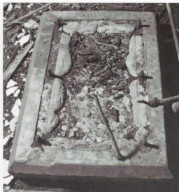
Photo 82. (Bottom center). Corroded metal reinforcing steel has caused significant spalling in ceiling of engine room area. The reinforced concrete ceiling is five feet thick at this point, so this spalling has not yet created any structural concern.
