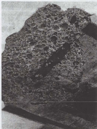
Embedded metal has caused spalling in the ceiling of Fort Columbia's mine casemate. Feb. 2008.
