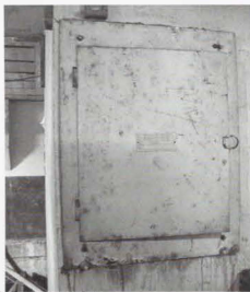
Photo 54. (Right). Original electrical box located west of door into casemate operating room.
