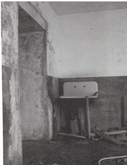
Photo 75. (Above). Battery room sink on east wall of casemate. Concrete infill above door from 1943 tunnel addition is shown. Repainting the casemate is not recommended based on the desire to preserve historic finishes. Although the interior of the 1921 casemate was painted, the 1941-43 addition appears to have received a plastered finish. Additional testing is necessary to determine the exact nature of the finishes.
