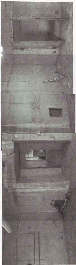
Photos 21-30. Ten photo sequence stitched to show 360 degree view of plotting room interior.
