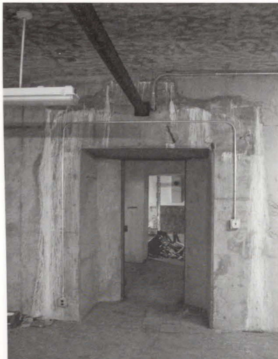
Photo 31. (Above). South doorway between plotting room and gas-proofing room. Note series of cold joints around the top of the door and severe efflorescence. Wall of plotting room is one foot thick here, added to three foot wall of gas-proofing room.
