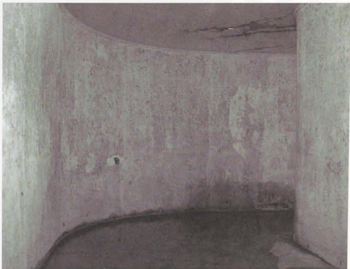
Photo 7. (Right). The second turn in the west entry tunnel. Note the very wet conditions at this point in the tunnel. Water was about 1/2" deep in February of 2008. Water infiltration seem to be predominantly from the significant crack system on the inside of the turn. This is one of the few structurally significant problem areas in the casemate. The concrete ceiling in this spot is about 1' thick, not as substantial as the rest of the structure.
