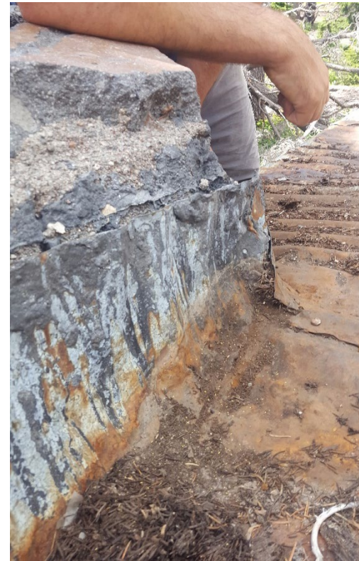
Failed seam at chimney
