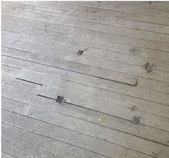
Typical construction and condition, absent Fire Finder
