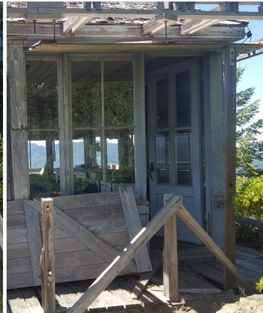
Altered northeast railing
