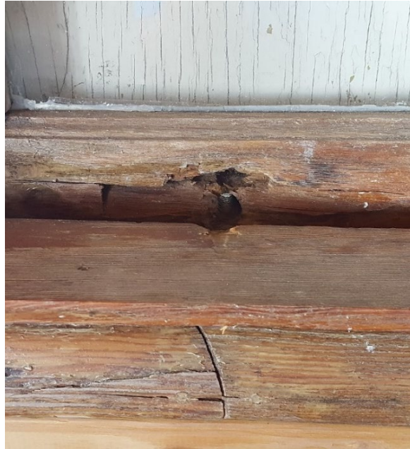
Condition caused by eyebolt installed through sash
