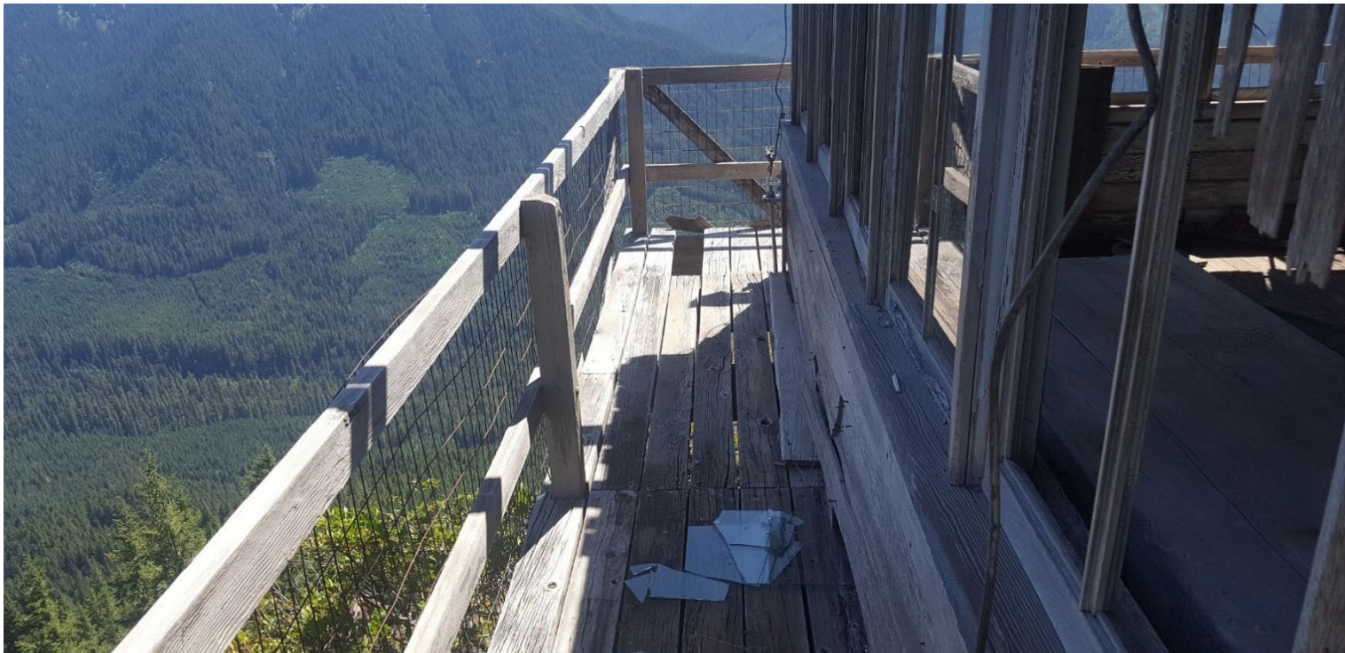
Weathered catwalk, broken glass, and broken windows on the southeast elevation
