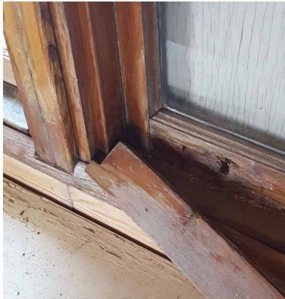
Window sill condition
