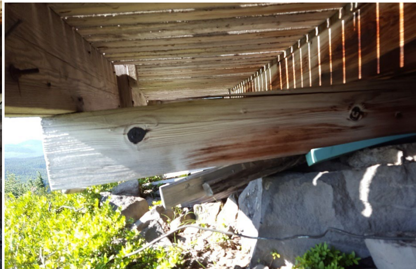
Cracked joist below east side catwalk
