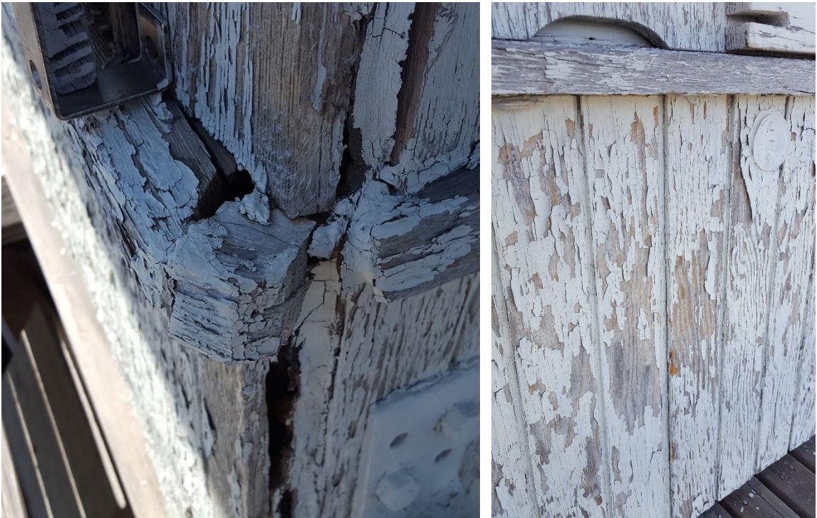
Figure 8. Photos of specific damage versus typical conditions
