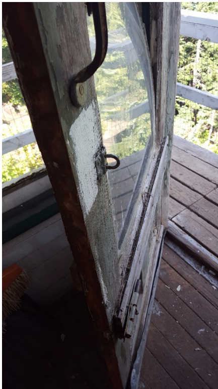
Typical condition, door
