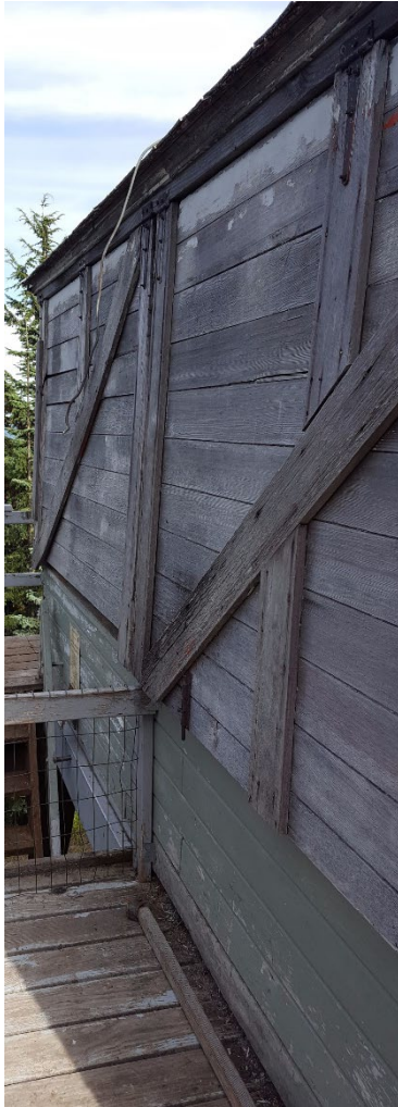
Condition of north shutters
