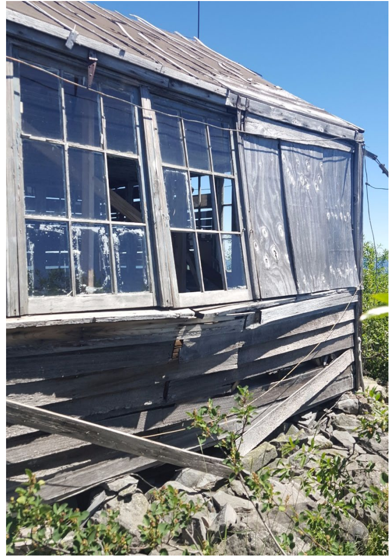
West wall condition
