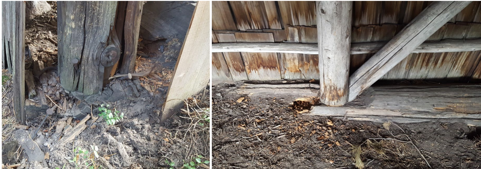
Typical condition of sills and posts demonstrated by the northeast corner and the rear wall
