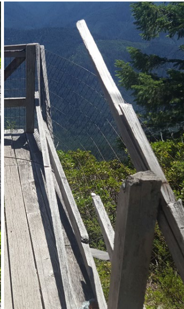
Broken northwest railing
