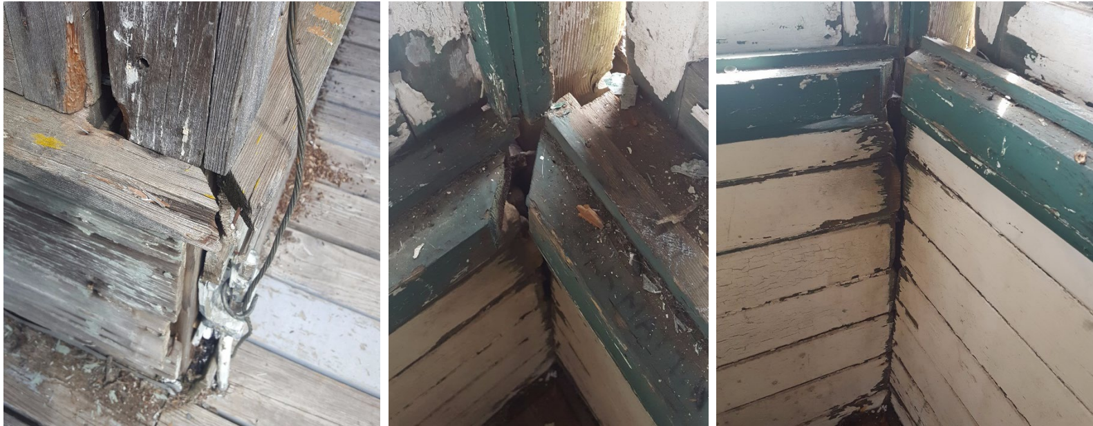
Separation of the south and west walls
