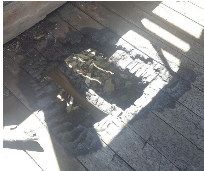
Burn damage (2' x 2')
