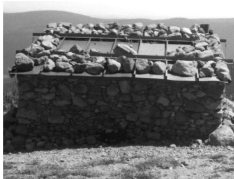
Rear wall condition, 1978. Courtesy of USFS
