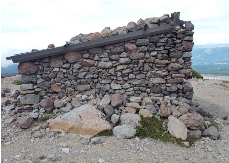
South wall condition and vertical crack, 2017
