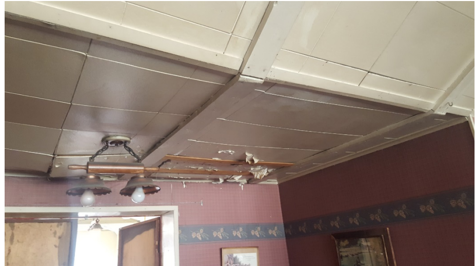
Dining hall ceiling condition
