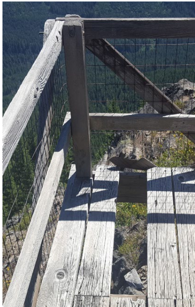
Missing deck boards, south corner
