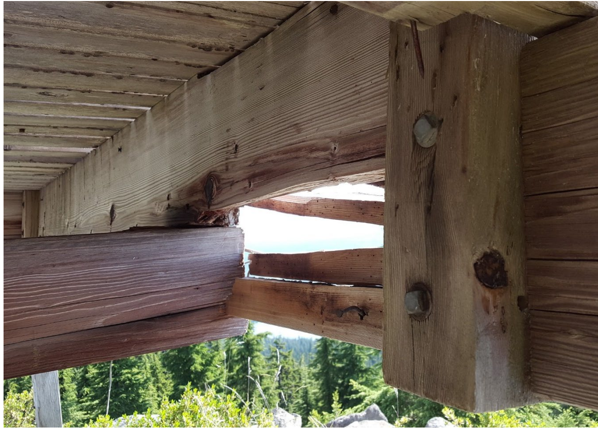
Damaged section of the catwalk on the east elevation
