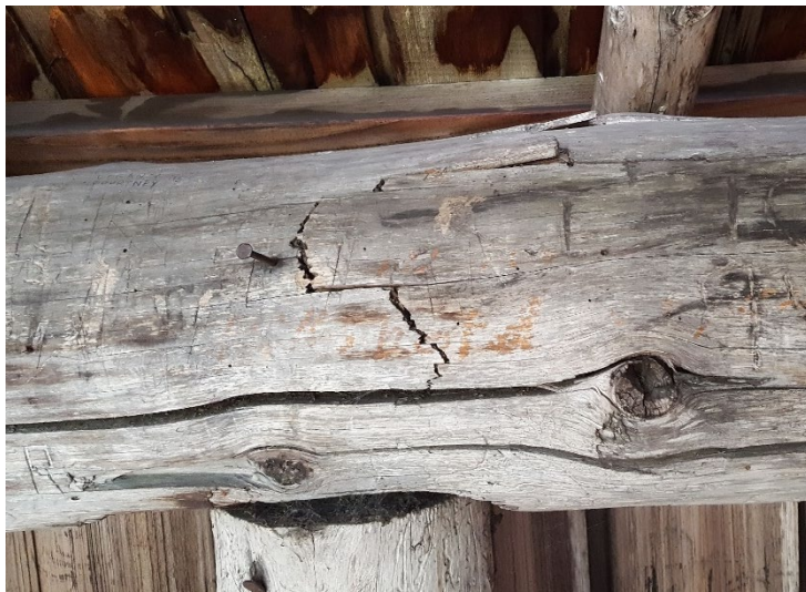
Condition of cracked rear beam
