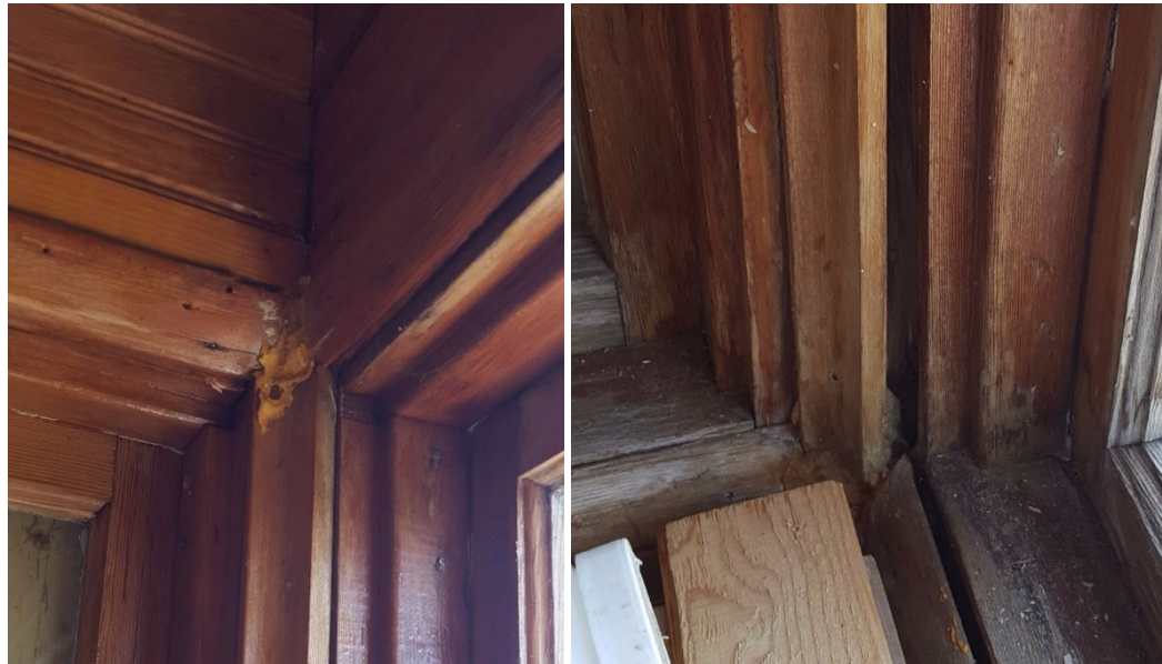
Trim and wall condition at the southeast corner
