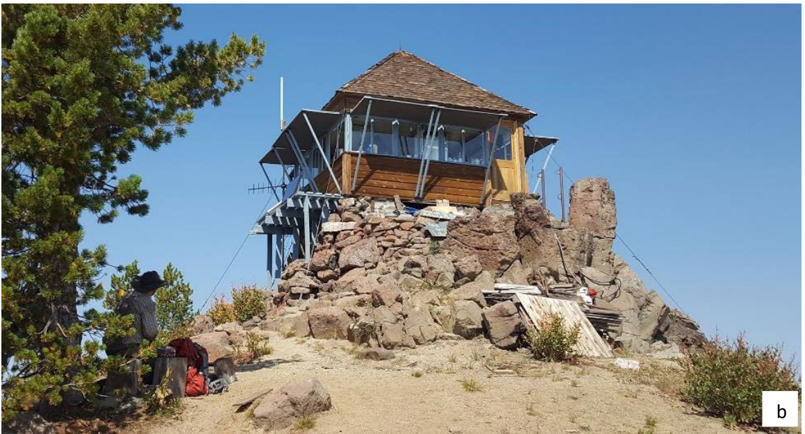
Figure 5.6. Preservation opportunities represented by (a) Olallie Mountain Lookout, which is in poor condition but retains integrity, versus (b) Mule Peak Lookout which is in good condition but has sustained some losses to integrity.
