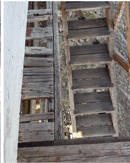
Deck condition, east side
