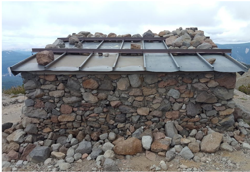
Rear wall condition and missing stones, 2017
