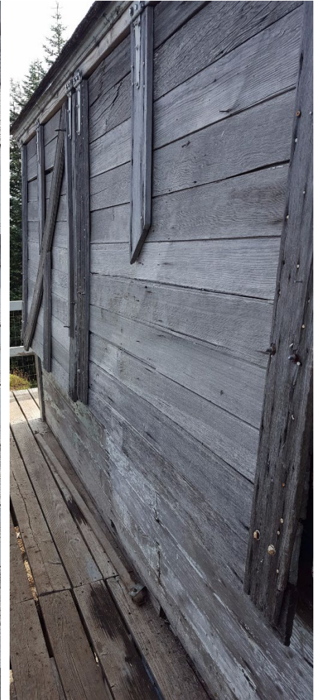
Condition of east shutters
