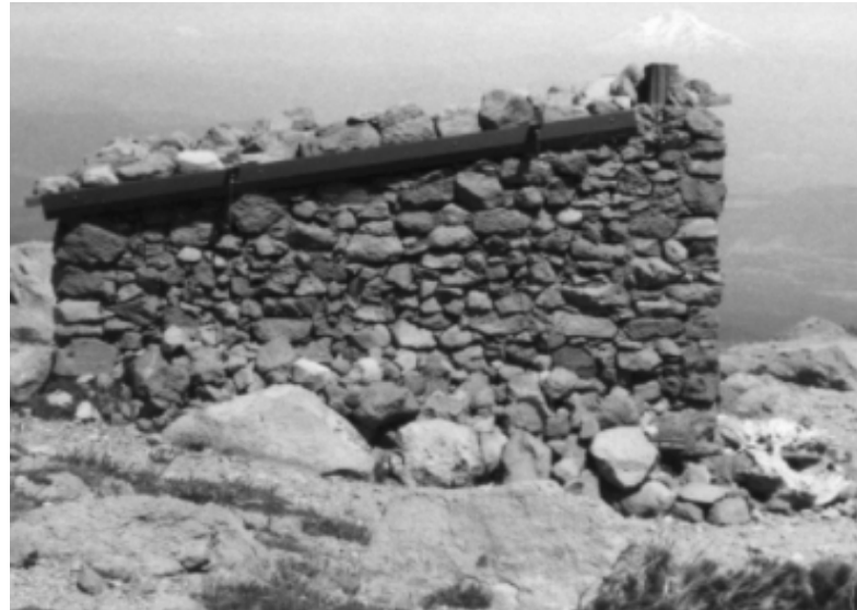
South wall condition, 1978. Courtesy of USFS
