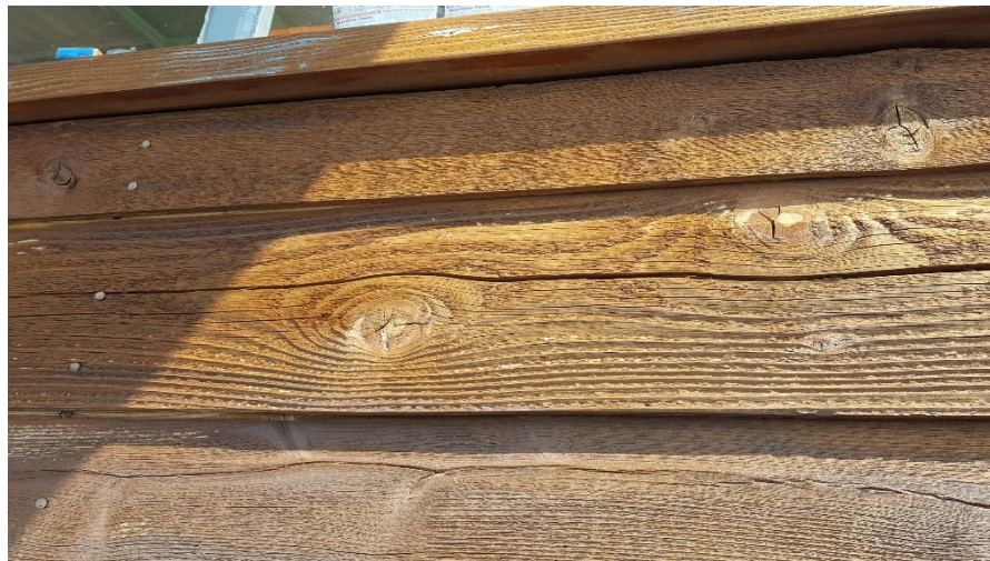
Typical condition of shiplap siding
