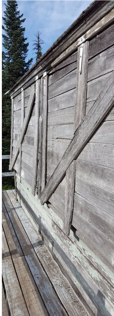
Condition of the west shutters
