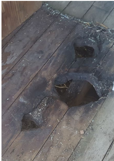
Burn damage (1' x 3')
