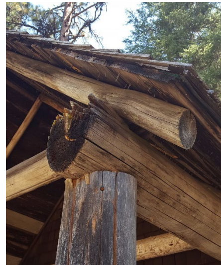
Condition at southwest corner
