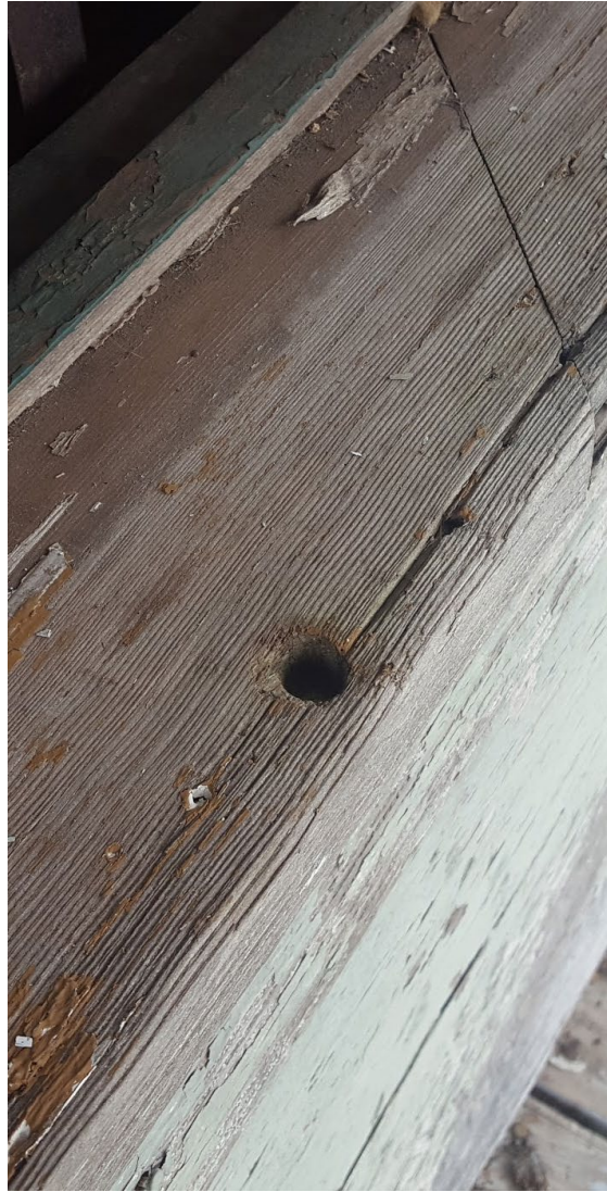
Typical condition, window sills
