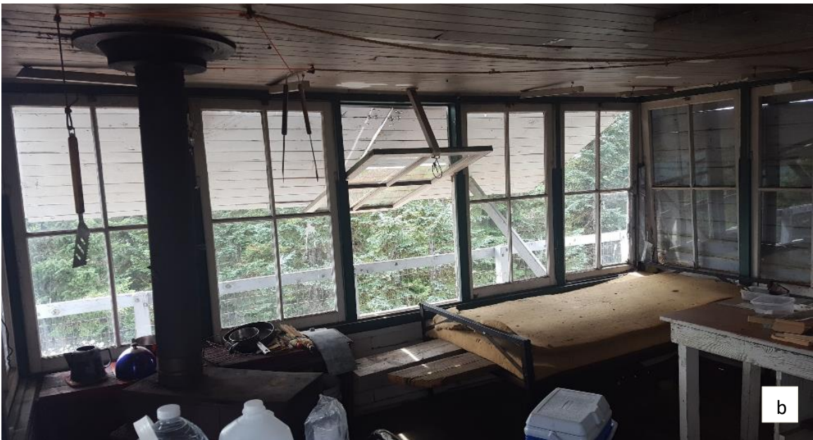
Figure 5.2. Exterior (a) and interior (b) views of Devil's Peak Lookout in the Salmon-Huckleberry Wilderness, Mount Hood National Forest in July 2017. This building exemplifies the effect of no administrative use and improvised maintenance on condition.
