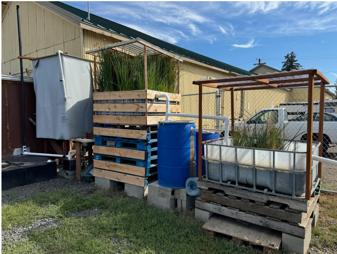
Figure 6: Graywater filtration system at a CSS site in Eugene (2024)
