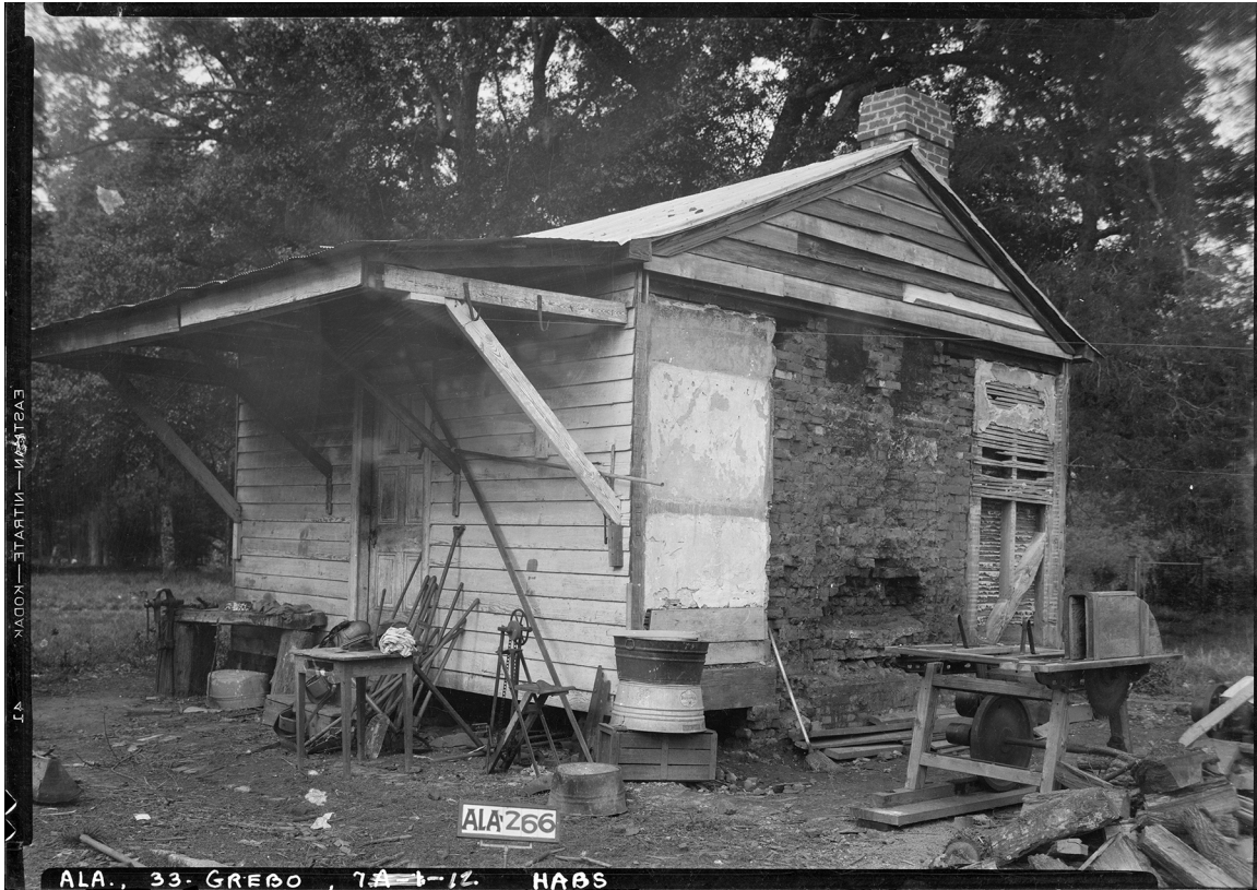
Fig. 30. Stud framed slave house in Hale County, Alabama demonstrating poor living conditions. By the 1930s, it was being used, apparently, as a blacksmithing and woodworking shop under the porch. Library of Congress, Prints & Photographs Division, HABS AL-266.
