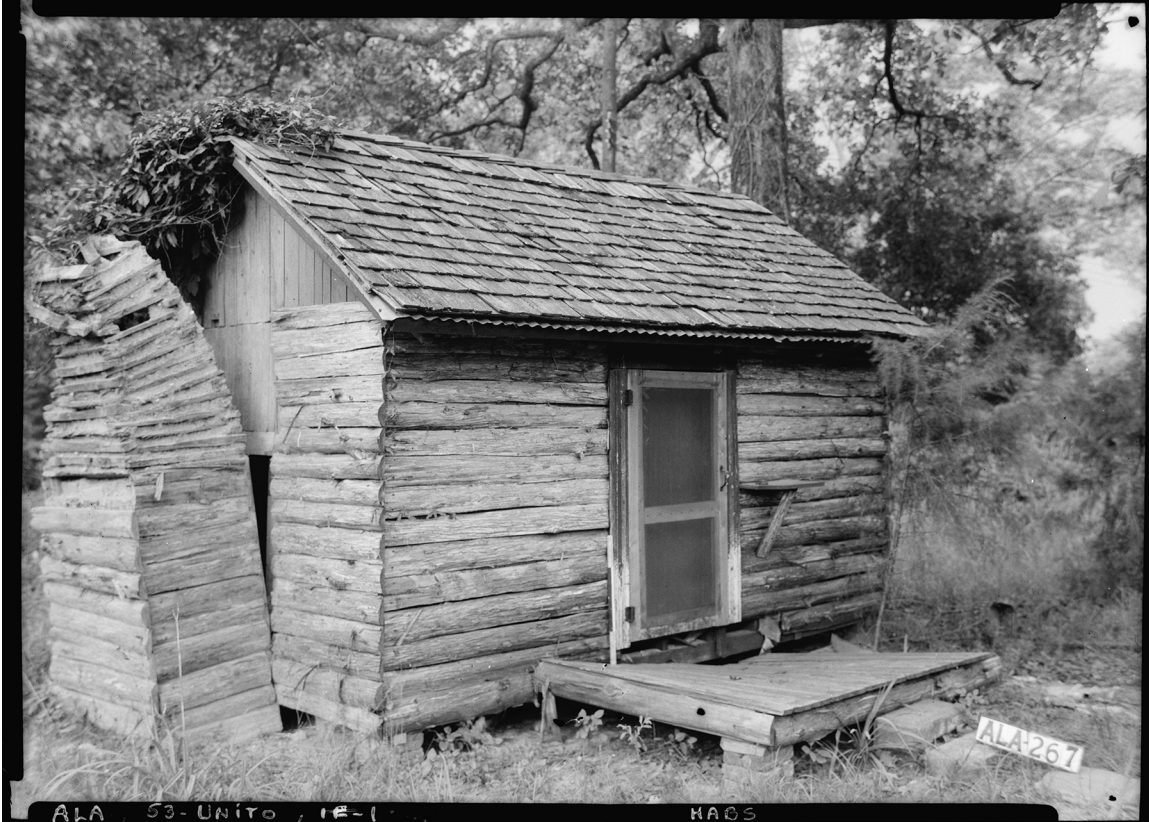
Fig. 27. Detail of catted chimney pulling away from the hearth from a slave house in Perry County, Alabama. The slave house is constructed from log slabs nailed to a stud framing system. Library of Congress, Prints & Photographs Division, HABS AL-267.
