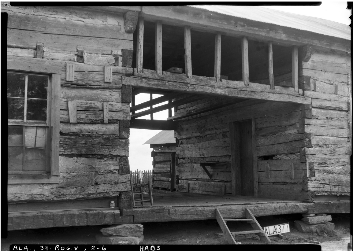
Fig. 44. Photograph showing windows with panes of glass at the first Taylor-Cunningham House. Library of Congress, Prints & Photographs Division, HABS AL-377-A.
