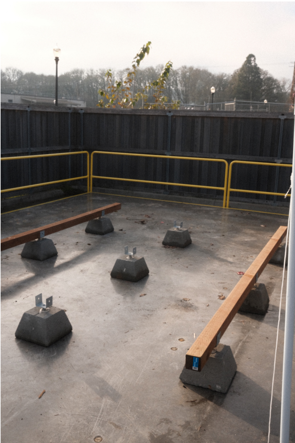
FIG. 42 The foundation of concrete piers and 4x4 lumber used for the build.
