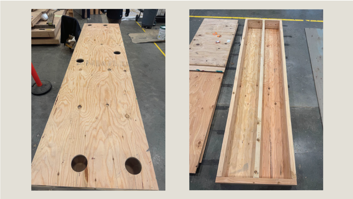
FIG. 28 The final two-foot by eight-foot wall with interior skin (left) and without interior skin (right).
